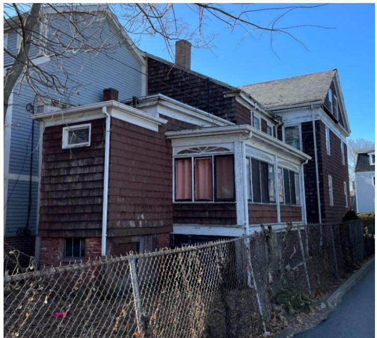
1899 one-story Baldwin addition and bathroom with enclosed porch added by a later owner.
