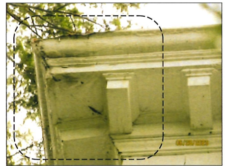
PHOTO #4 WD-COR-01: REMOVE DETERIORATED CORNICE CORNER AND REPLACE TO MATCH EXISTING. REPAIR ANY UNDERLYING STRUCTURAL DETERIORATION USING APPROVED UNIT PRICES. PREPARE, PRIME AND PAINT.
