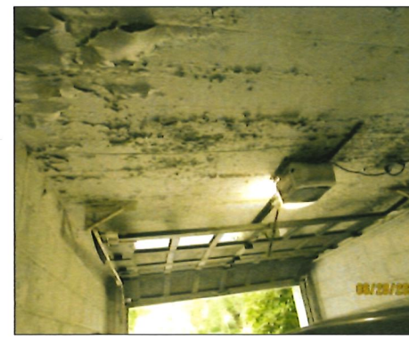
PHOTO #10 PT-MAS-02: REMOVE PEELING PAINT. REPAIR CONCRETE SLAB UNDERSIDE. PREPARE, PRIME AND PAINT INTERIOR CMU WALLS AND CONCRETE CEILING. PAINT INTERIOR AND EXTERIOR OF THE GARAGE DOOR.
