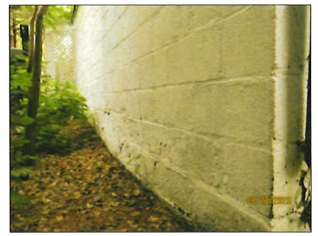
PHOTO #8 PT-MAS-02: REMOVE AND REPLACE CMU AS REQUIRED. PREPARE, PRIME AND PAINT EXTERIOR CMU WITH A BREATHABLE MASONRY COATING (ASSUME 100%).
