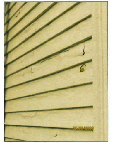
PHOTO #9 PT-SID-01: USING APPROPRIATE LBP SAFE MEASURES, REMOVE PEELING PAINT. PREPARE, PRIME AND PAINT EXTERIOR WOOD (ASSUME 100%).
