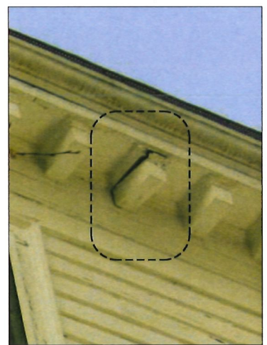
PHOTO #3 WD-COR-01: REMOVE DETERIORATED DENTIL AND REPAIR ANY UNDERLYING STRUCTURAL DETERIORATION USING APPROVED UNIT PRICES. REPLACE TO MATCH EXISTING. PREPARE, PRIME AND PAINT.
