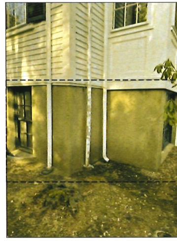
PHOTO #11 SU-FOW-01: REPAIR EXTERIOR PARGE COAT. APPLY NEW BREATHABLE COATING OVER EXTERIOR MASONRY WALL (ASSUME 100% COATING)
