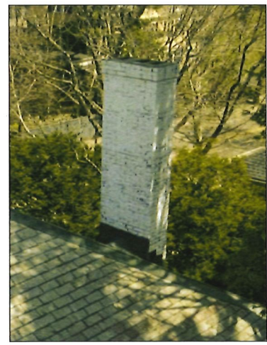
PHOTO #7 PT-MAS-01: REMOVE AND REPLACE BRICK MASONRY AS REQUIRED. REPOINT BRICK MASONRY AS REQUIRED (ASSUME 100%). REMOVE PEELING PAINT. PREPARE PRIME AND PAINT BRICK WITH A BREATHABLE MASONRY COATING. REPLACE SEALANT AT STEPPED FLASHING.
