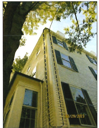
PHOTO #2 WD-SID-02 & MT-GUT-03: REMOVE WARPED WOOD TRIM AND REPLACE TO MATCH EXISTING. PREPARE, PRIME AND PAINT (ASSUME 100%).
