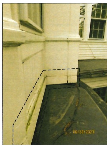
PHOTO #1 WD-SID-02 & MT-GUT-03: REMOVE DETERIORATED BASE TRIM, MOULDINGS AND PLINTHS, AND REPLACE TO MATCH EXISTING. PREPARE, PRIME AND PAINT.
