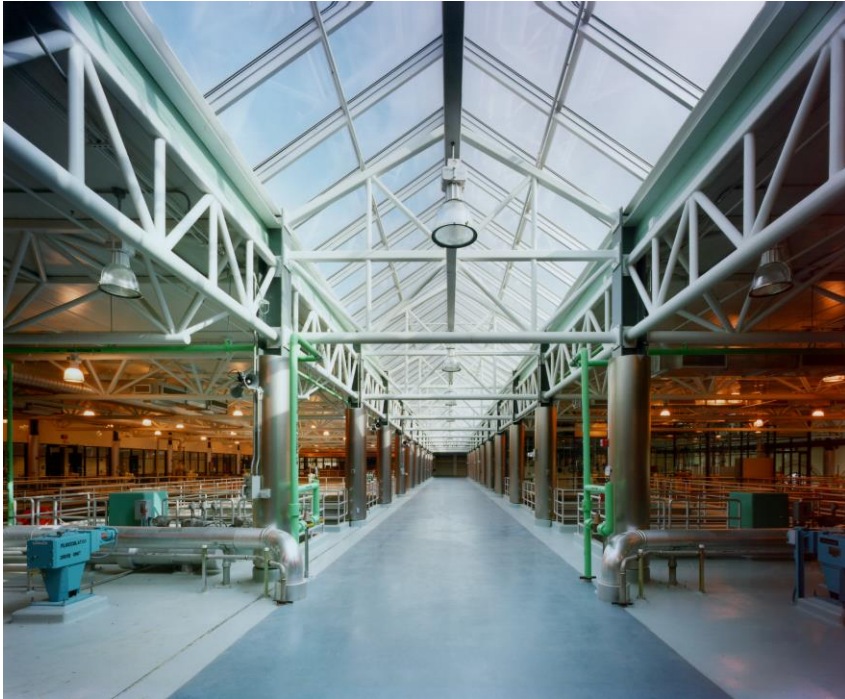
Main Process Floor
