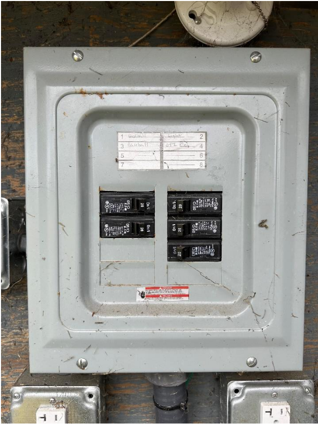
Electrical Cabinet Panel
