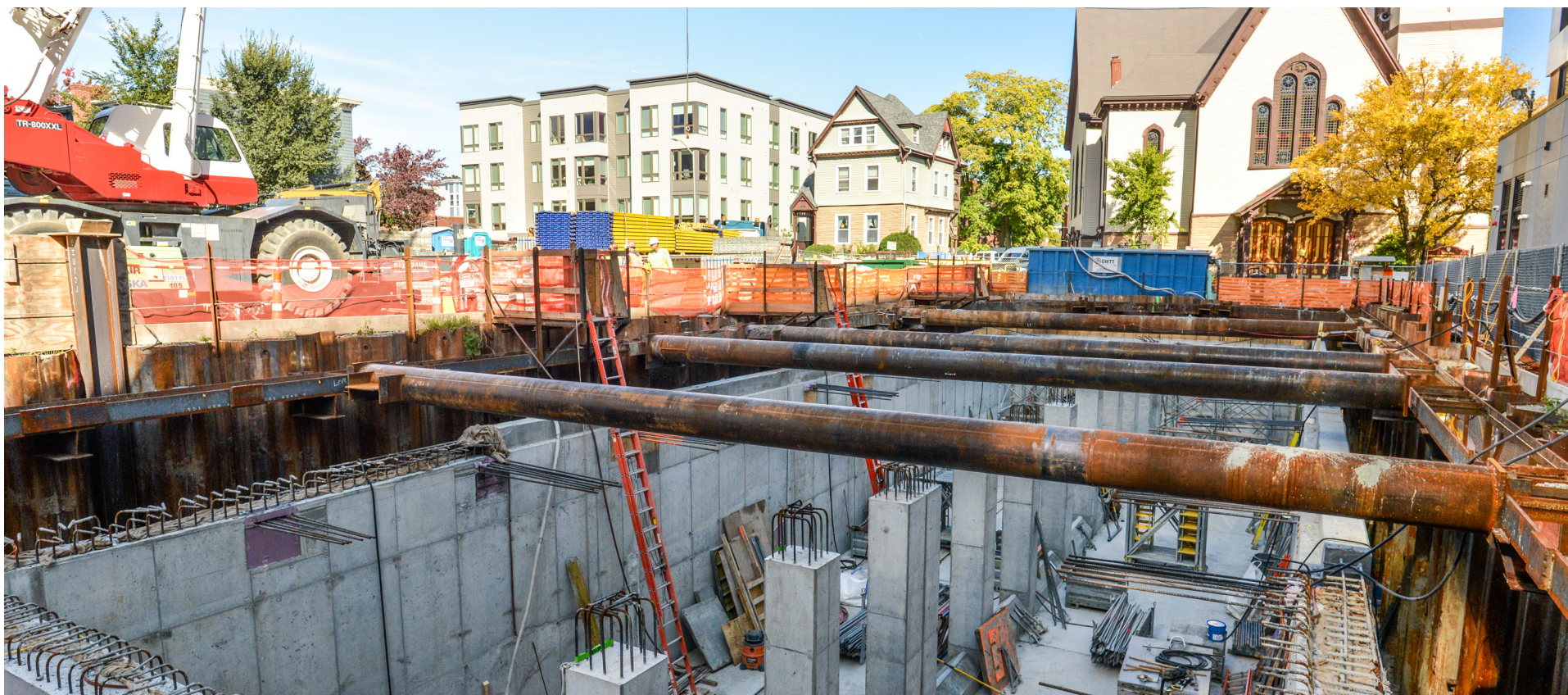
Figure 26. The construction of the PL6 tank in the Port is part of a comprehensive plan to capture excessive stormwater in the neighborhood during extreme weather events. Source: City of Cambridge, June 2020.
