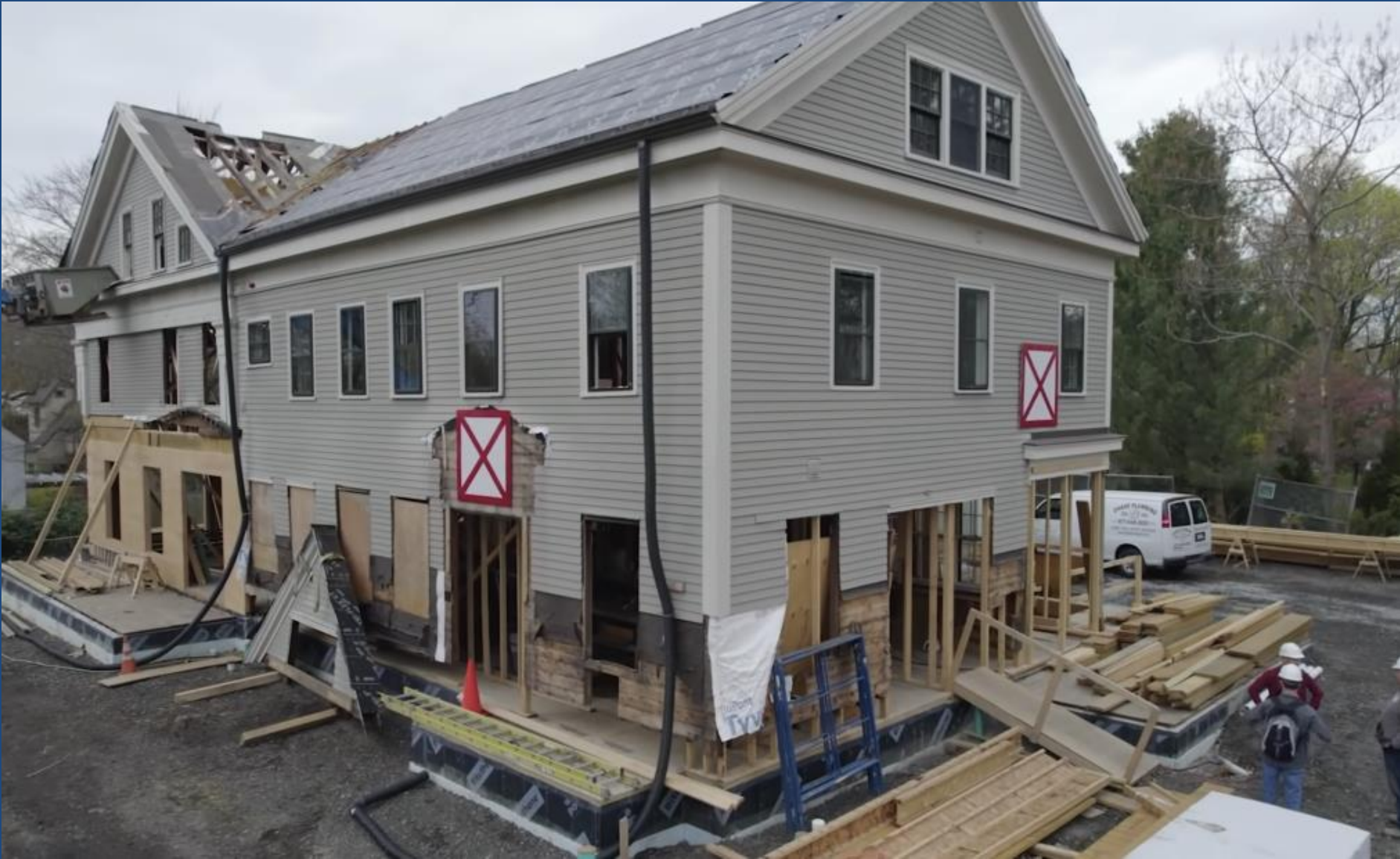
12 Lake View Avenue lowered on its new foundation, with original framing and exterior still in place, Spring 2022. Screenshot, The Bridge podcast
