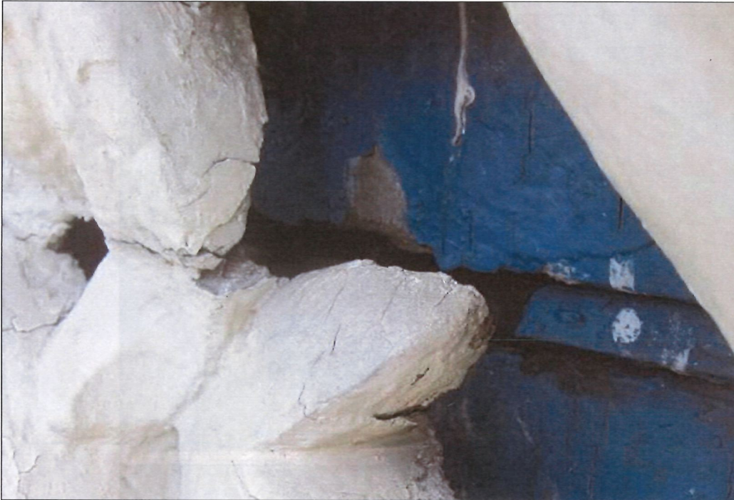
West backboards deteriorating and sections are missing
