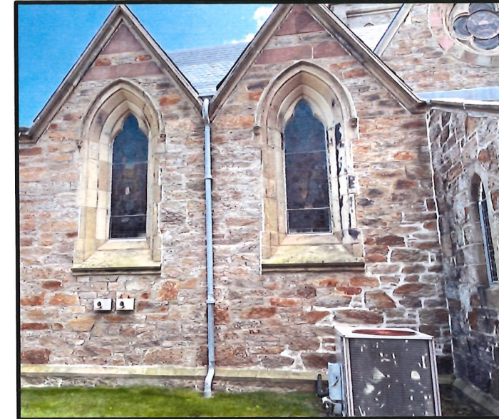
EXISTING HVAC EQUIPMENT
