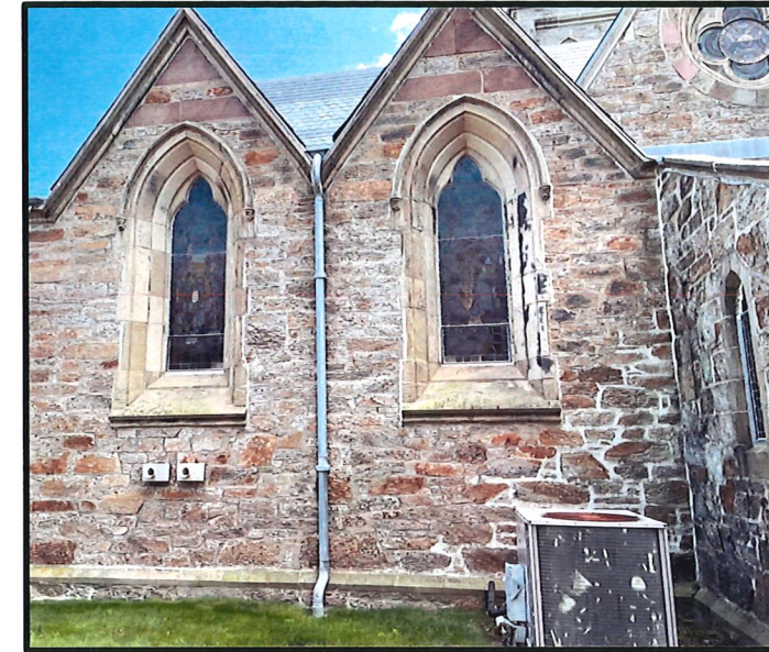
EXISTING HVAC EQUIPMENT
