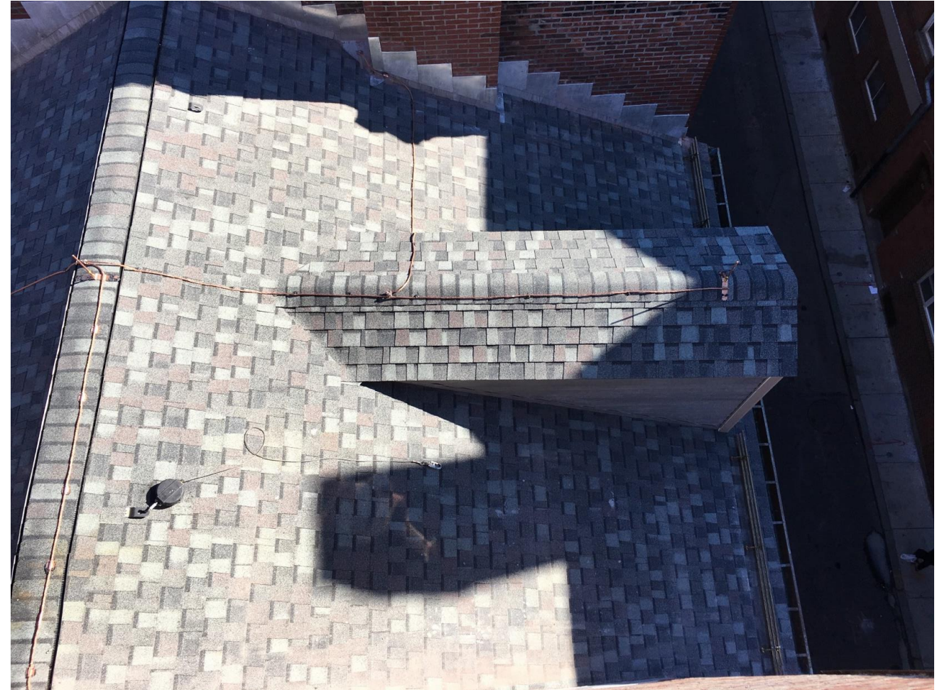
Example of Lightning Protection on Roof (Harvard University project provided by FAA)
