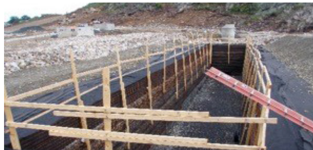
Figure 24. Underground infiltration basin under construction at the Waltham Polaroid redevelopment site [Source: Cambridge Water Department]
