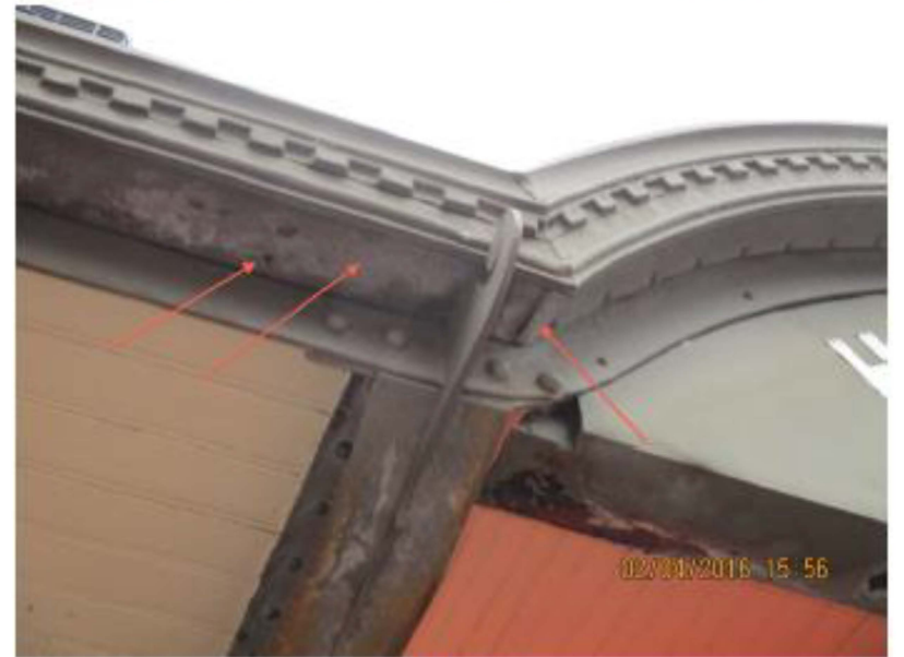
Photo 26 West elevation: Decorative cornice detail. Note accelerated oxidization of the lead coating.
