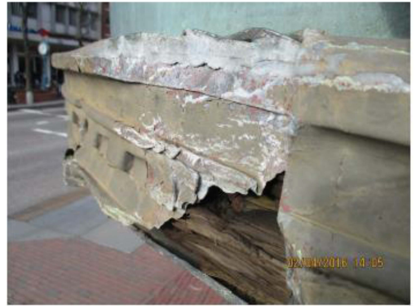
Photo 25 Southwest decorative cornice damage and wood blocking.
