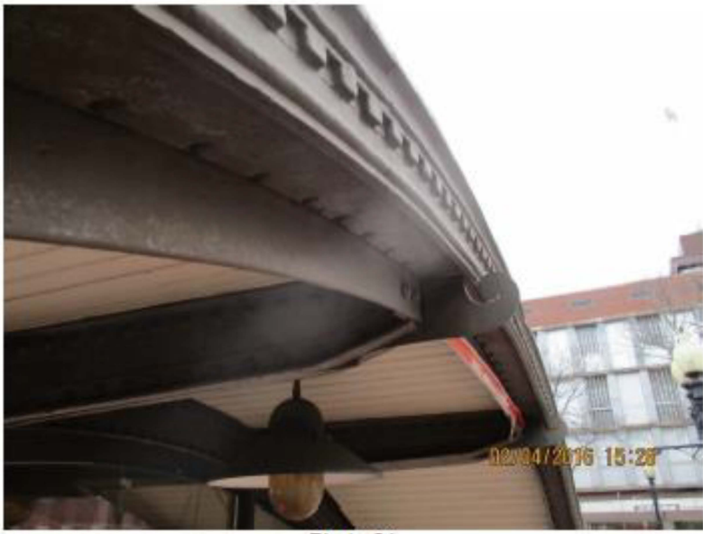
Photo 21 North elevation: Detail of decorative lead coated copper cornice and steel framing.
