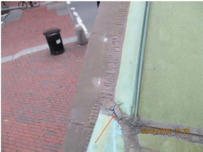
Photo 22 North elevation: Detail of transition between the standing seam copper roof and decorative cornice. Note failed solder joint.
