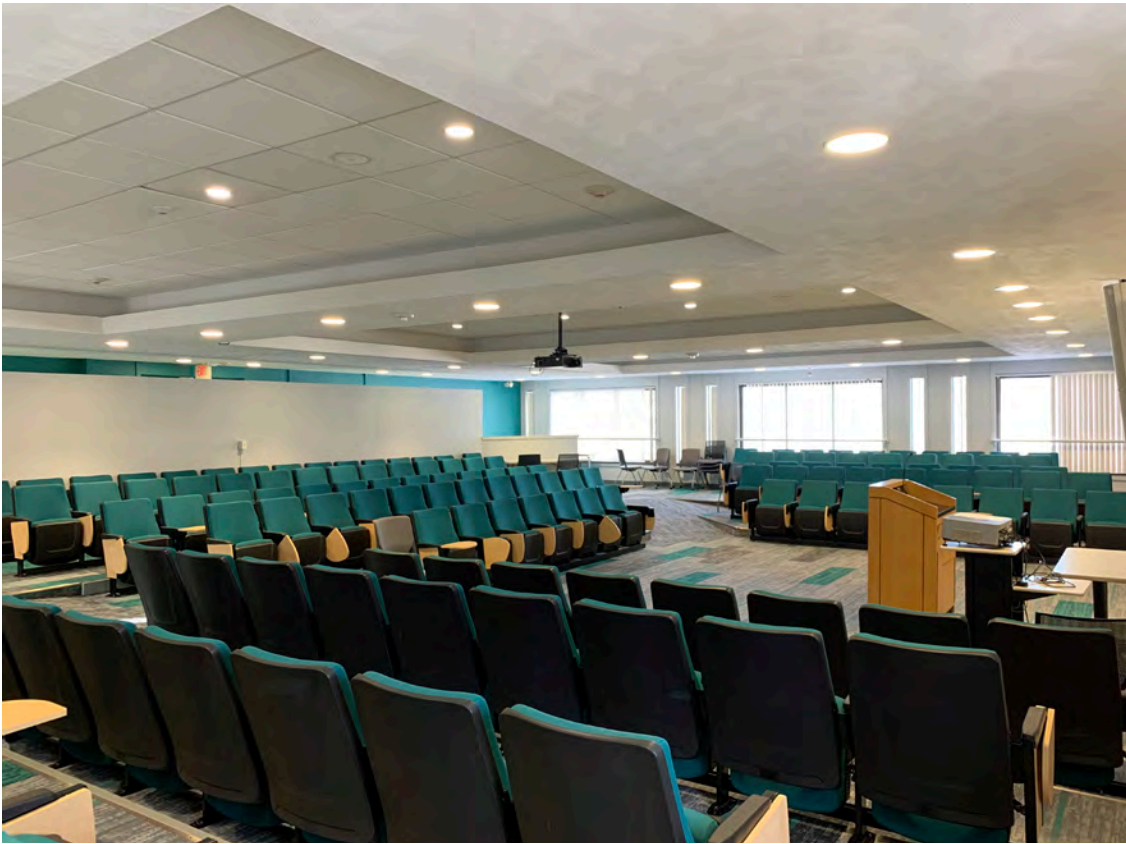
SHERRILL'S THIRD FLOOR CLASSROOM WAS RENOVATED TO PROVIDE THEATER-STYLE SEATING AND NEW FINISHES.
