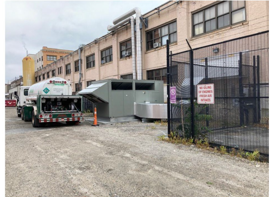
MIT Building Number NW12 Carbon Dioxide delivery photo
