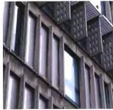
Precast concrete fins (south)
