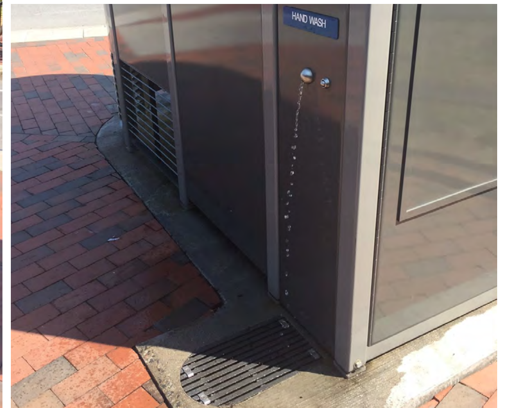
Hand Wash Station
