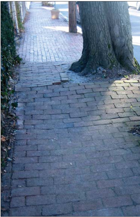
Figure 17. Original sandset brick sidewalk, uneven from root lift on Tremont Street in Area 4.
