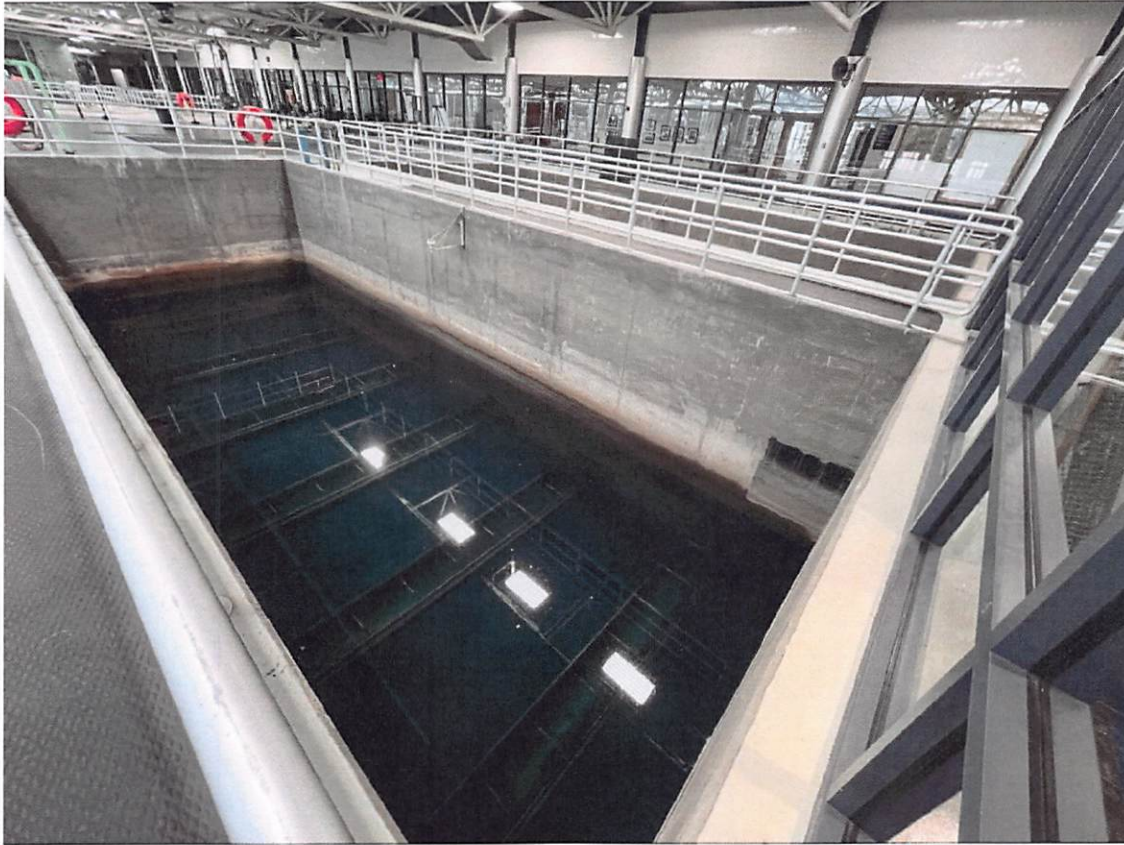
One of the water filters with newly replaced granular activated carbon media
