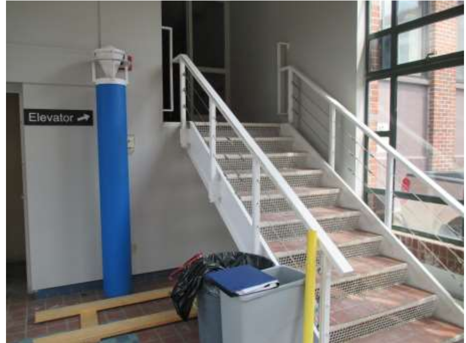
Existing first floor is approximately 5 feet above street level, which inhibits gathering and assembly uses
