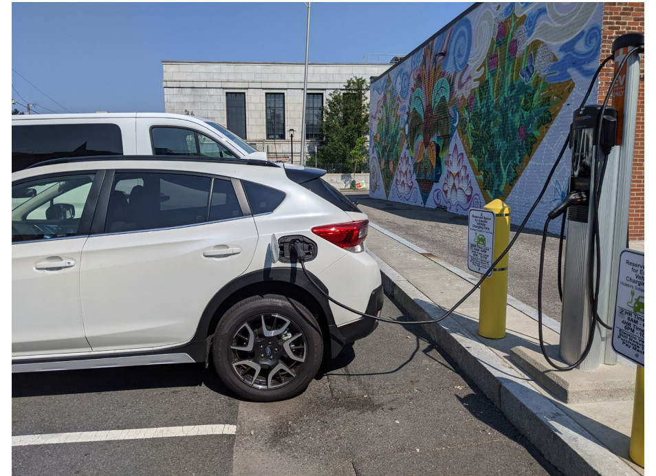
Lot 8 EV Charger
