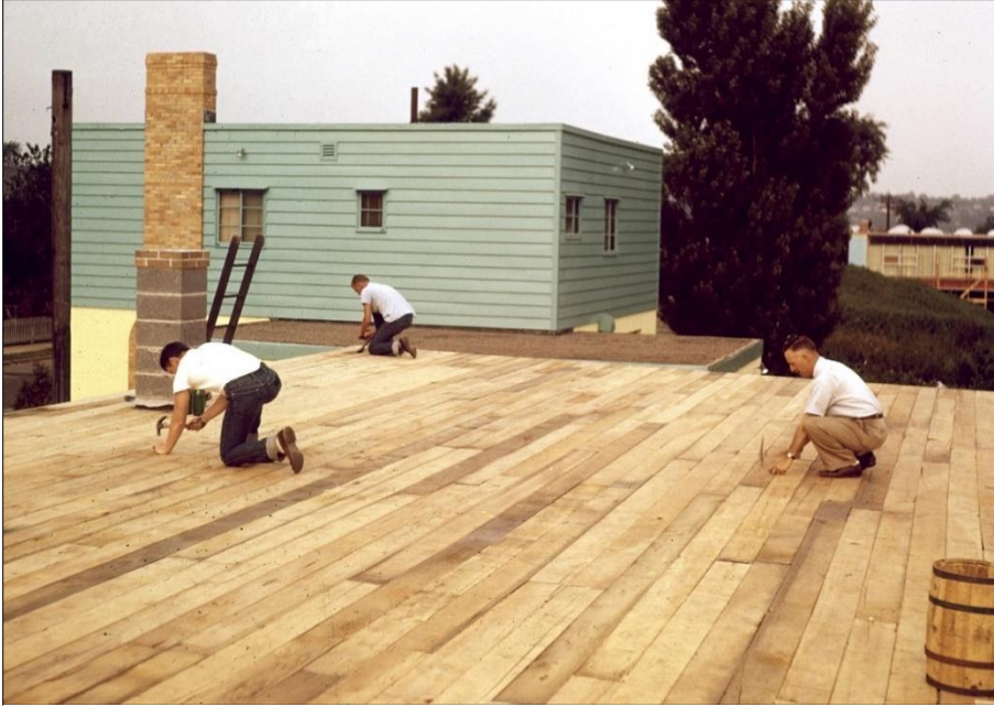
47-53 Bay State Road. Construction of one-story annex building, 1956, with Solberg house at rear. Photo courtesy of Sky & Telescope Magazine.
