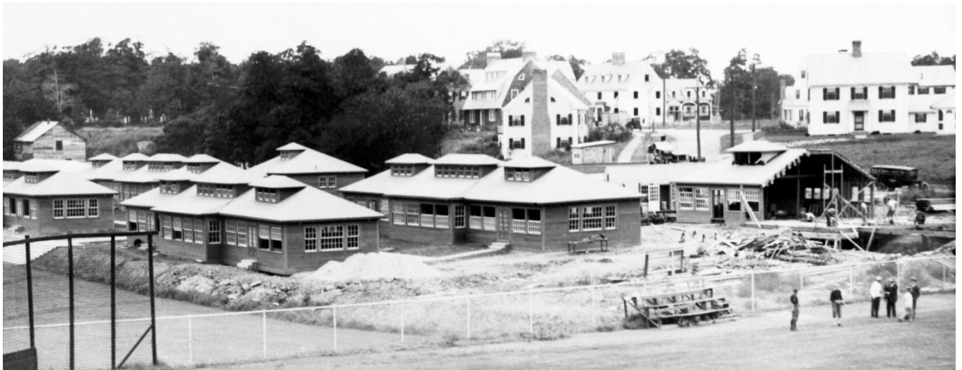
The new Shady Hill School under construction at Coolidge Hill. Photo ca. 1926.
