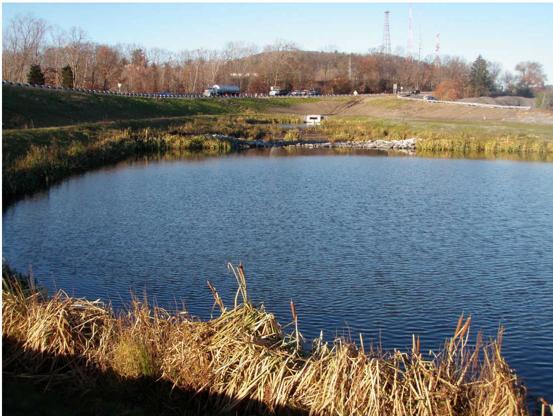
Figure 10. A , Construction of a structural source control—wet ponds separated by elevated gravel wetlands—in November 2011, B , bank erosion around the nearly completed structural source control in June 2012, and C , completed project, November 2012, upstream from U.S. Geological Survey continuous water-quality monitoring station 01104455 in the Cambridge drinking-water source area, Massachusetts. Photographs courtesy of David Kaplan, Cambridge Water Department, Massachusetts. Location of station is shown in figure 1.
