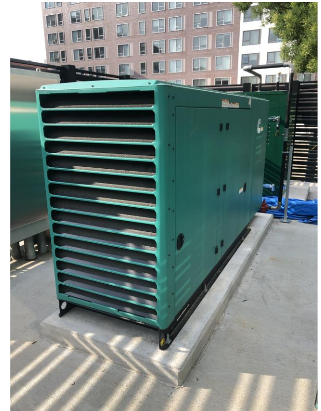
Generator for PL6 Stormwater Tank.
