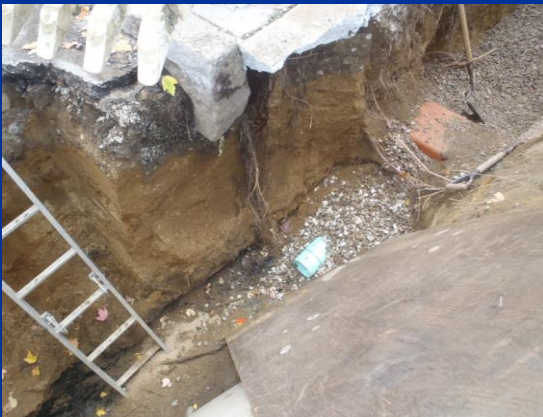
Ladder too short
