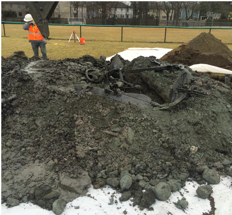
-Stockpile of waste fill material showing metal car frame removed at approximately 11' bgs.
