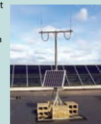
Rooftop receiving unit for daily readings from customers' meters.
