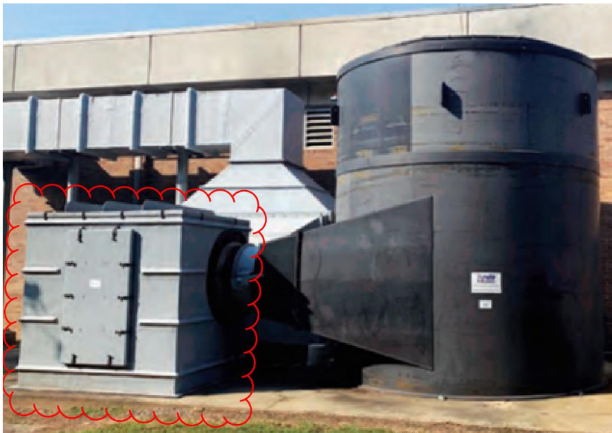
Figure 3-23. Dedicated Fan and Motor Acoustic Enclosure
