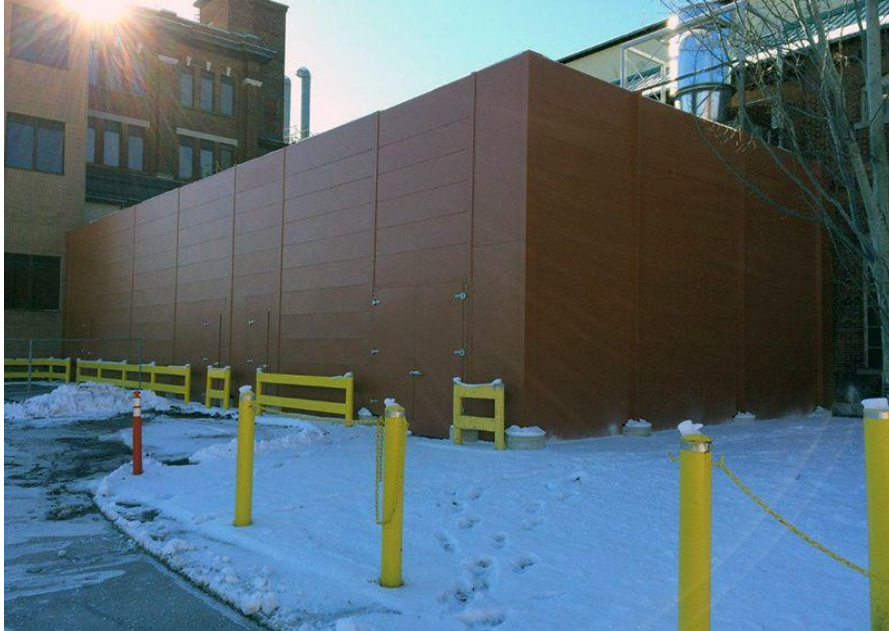
Figure 3-22. Perimeter Acoustic Panel Enclosure Example
