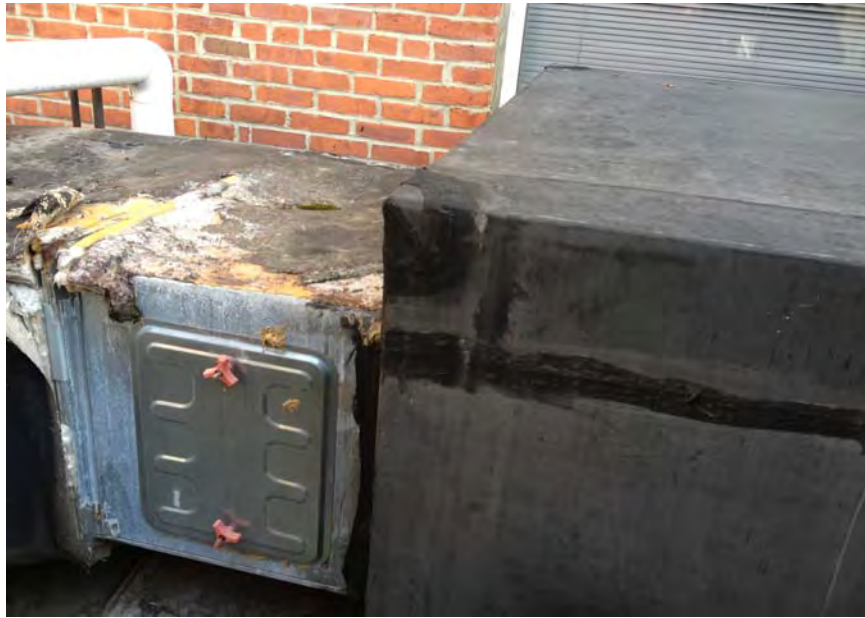
Image 17: Return ductwork at roof plenum box
