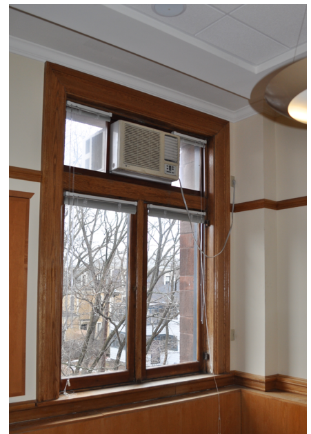
Fig. 307 - Existing AC unit
