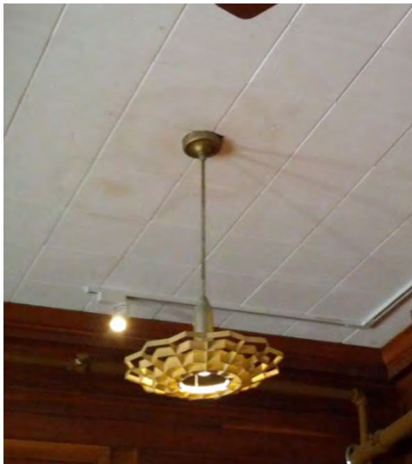
Water damage to acoustical ceiling tiles
