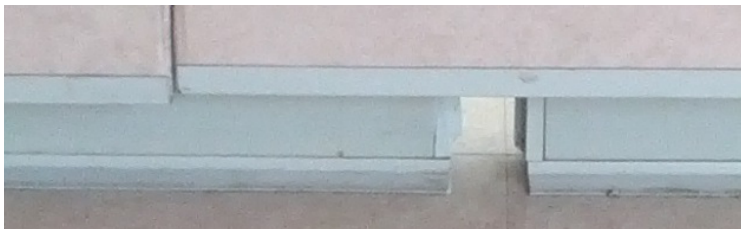
Fig. 411 - Gaps in operable partition at floor level
