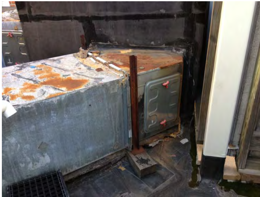
Image 16: Supply ductwork along the roof
