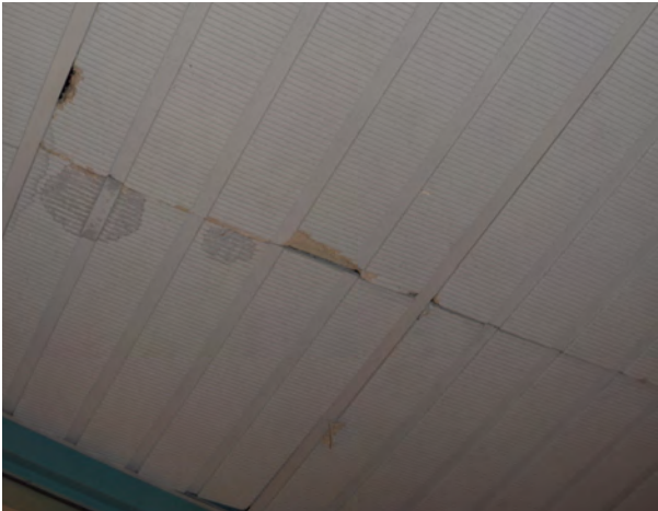
Fig. 402 - Stained/damaged acoustic ceiling tile
