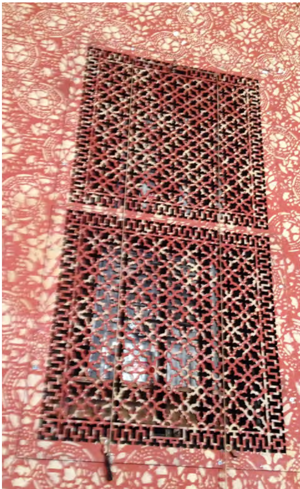
Fig. 126 - Existing electric heaters behind metal grille
