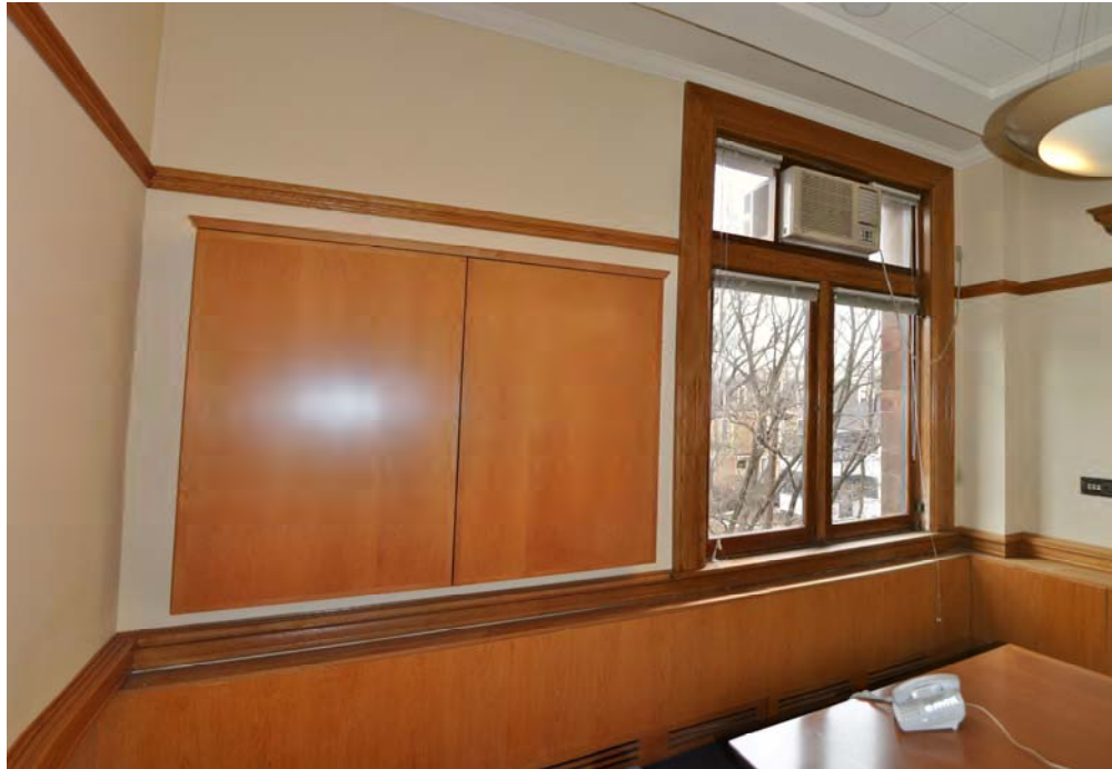
Image 7: Window Air Conditioning Unit
