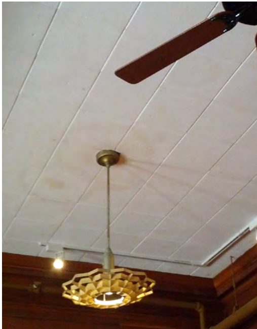
Fig. 206 - Existing ceiling fan, pendant & track lighting (note damaged acoustic tile)
