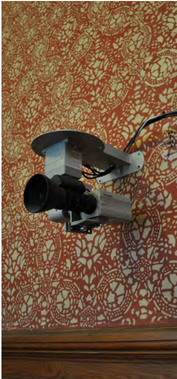
Fig. 105 - Existing Video Camera
