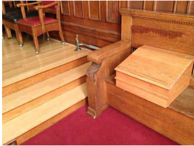
Image 5: Piping along front wall at platform
