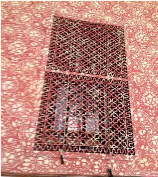
Image 1: Wall grille with fan heaters
