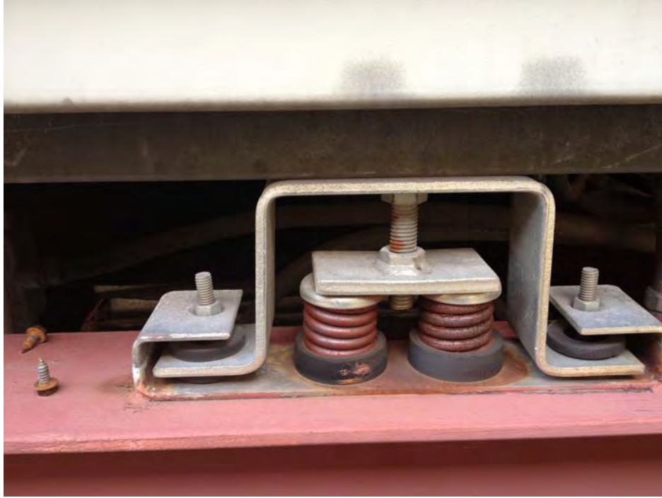
Image 15: Typical spring isolator at the rooftop unit
