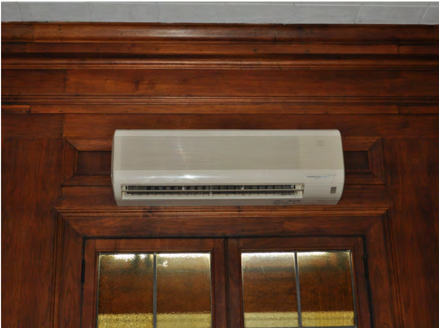
Fig 205 - Existing split system unit
