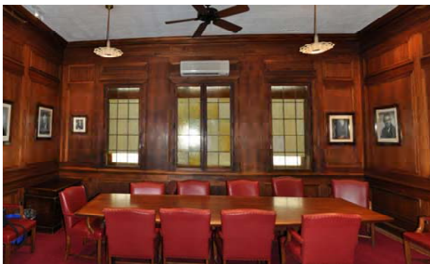
Image 9: Existing Ductless Split System
