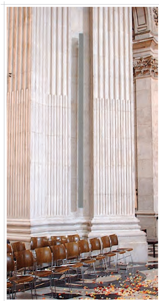
An Intellivox-DS500 installed at St Pauls Cathedral, London, UK
