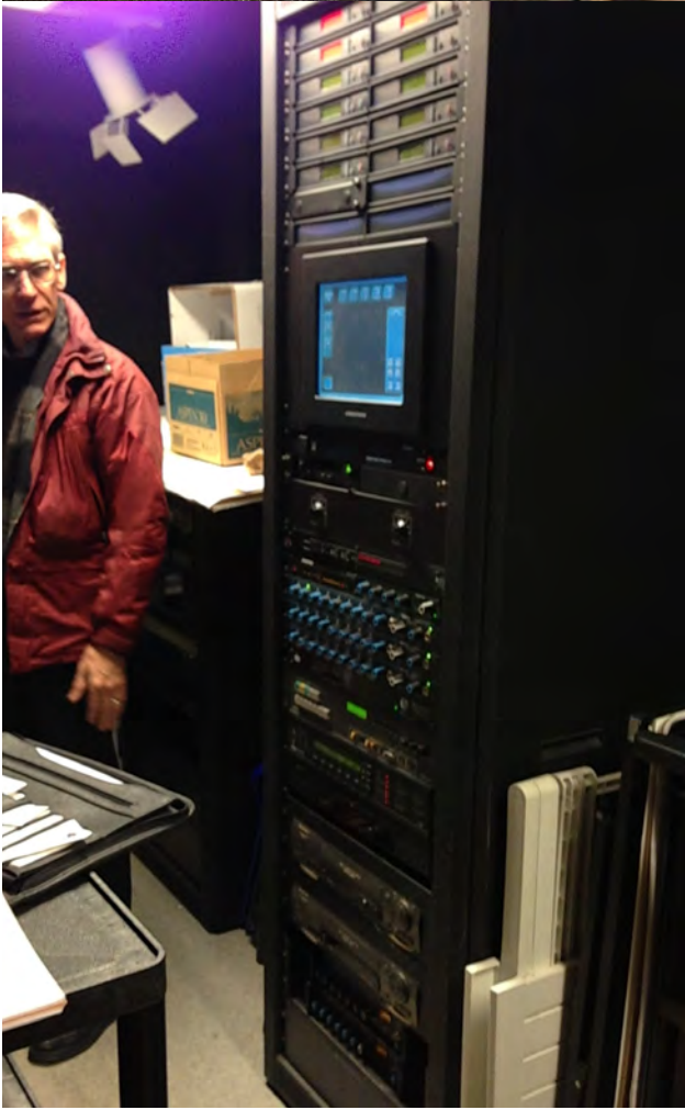
Fig. 505 - Existing audiovisual equipment
