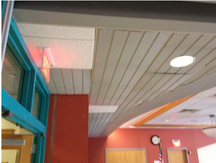
Image 13: Dropped ceiling used for return air
