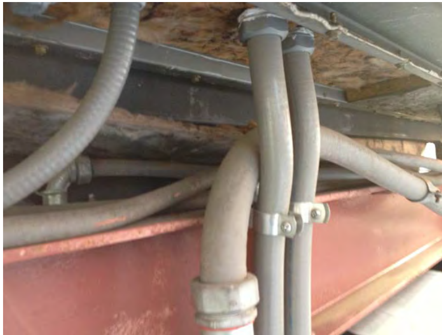
Image 18: Electrical connections at the rooftop unit
