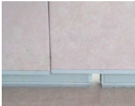
Clear gap at the bottom of the operable partition.
