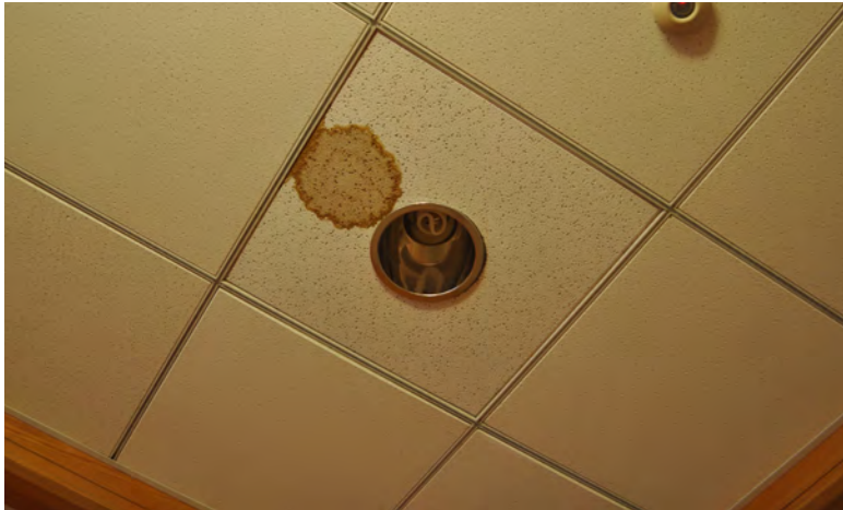
Fig. 401 - Stained/damaged acoustic ceiling tile
