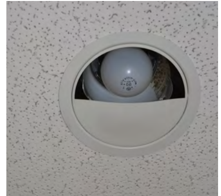
Fig. 706 - Existing incandescent lamp
