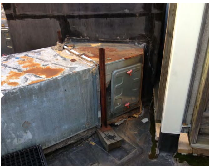
Fig. 417. Uninsulated, deteriorating ductwork at rooftop equipment
