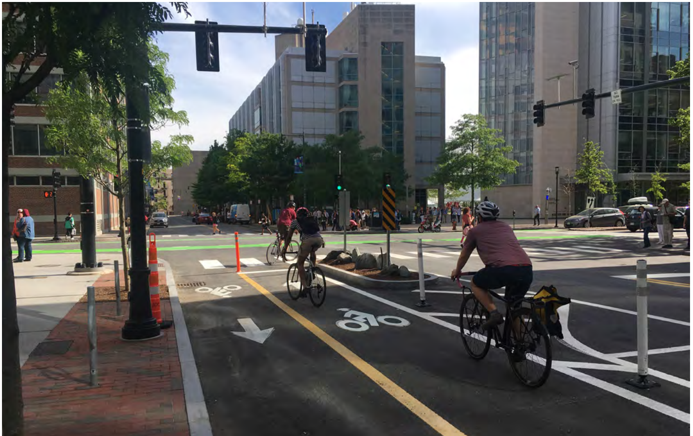
This two-way separated bike lane on Ames Street uses traditional construction and quick-build materials.
