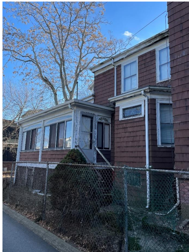
View of 1899 addition; 1900 bay window added by Louis F. Baldwin and enclosed porch by a later owner.
