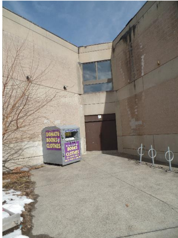
Photo 11: Exterior Masonry Wall - Moisture Damage
