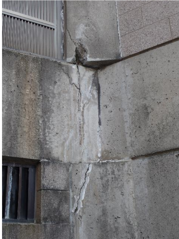
Photo 7: Corrosion/Spalled Concrete Cover and Cracking/Deterioration
