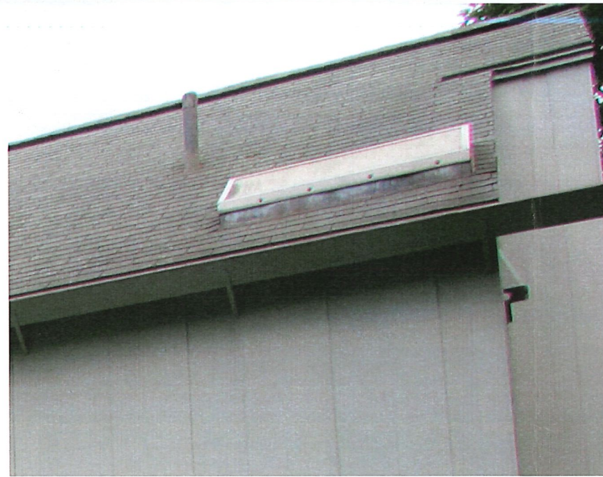
Existing Condition at Skylight (does not match drawing)
