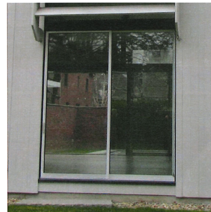
Existing Condition At Sliders
