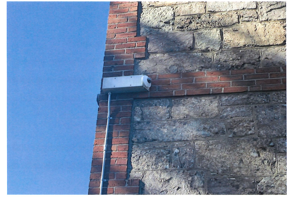
Burnham Hall Facade mounted security camera - wi-fi
