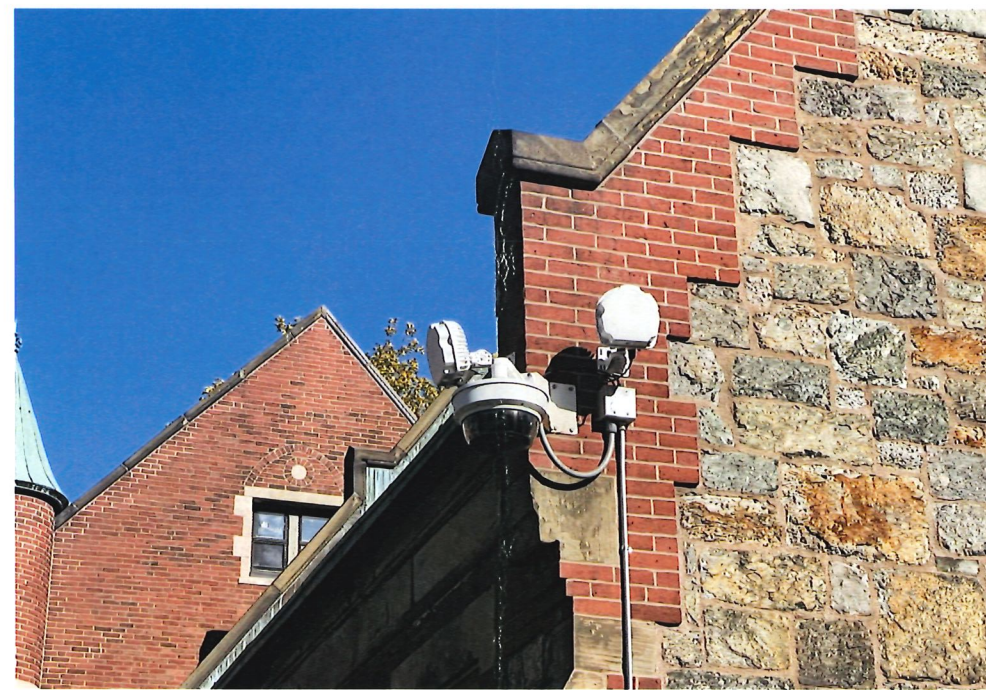
Burnham Hall Facade mounted security camera - wi-fi
