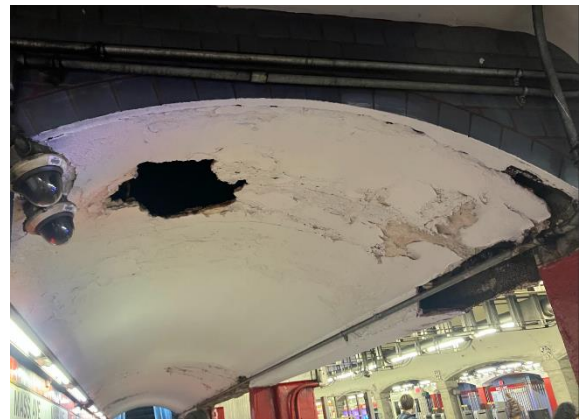
1: Hole in ceiling of station exit.
