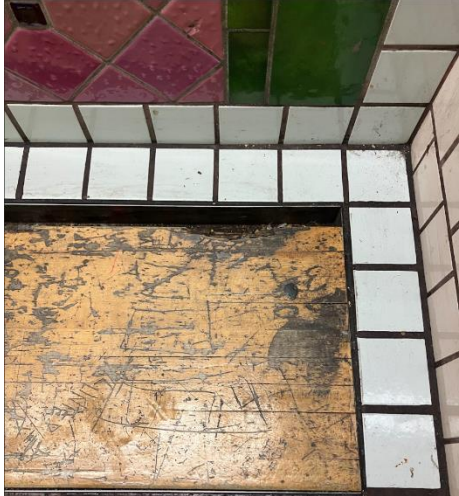
2: Bench missing plank of wood
