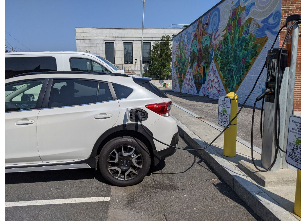
Lot 8 EV Charger
