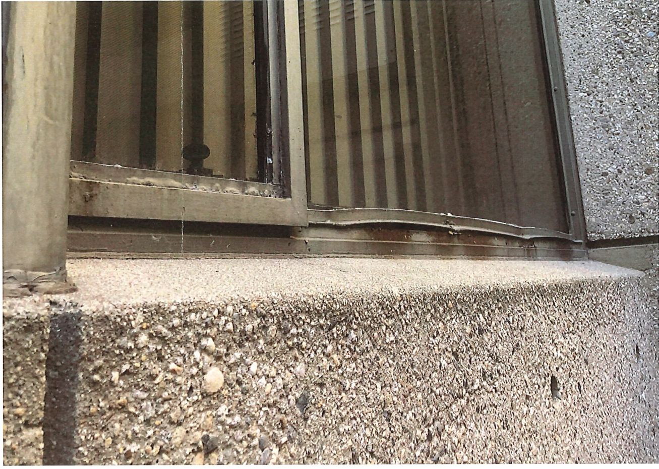
Warping and rusting of frame and sash at base of fixed window
