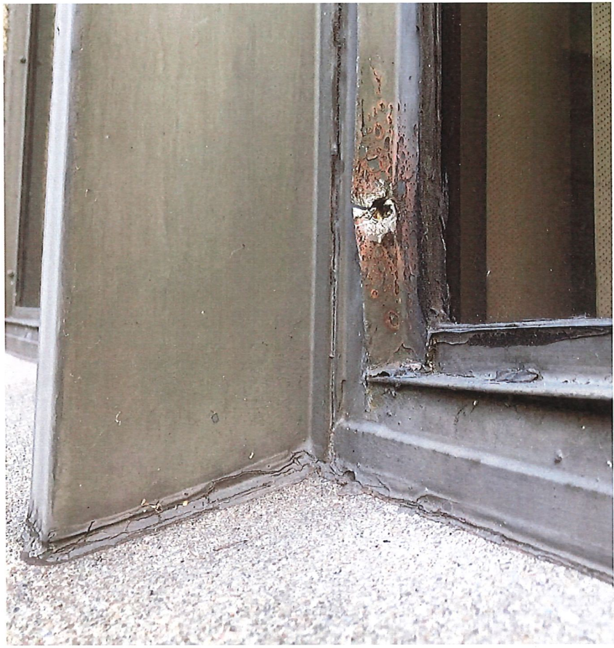
Missing fastener and rusted hole at sash connection
