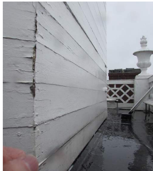
WOOD SIDING AT LOWER TOWER SECTIONS IN POOR CONDITION
