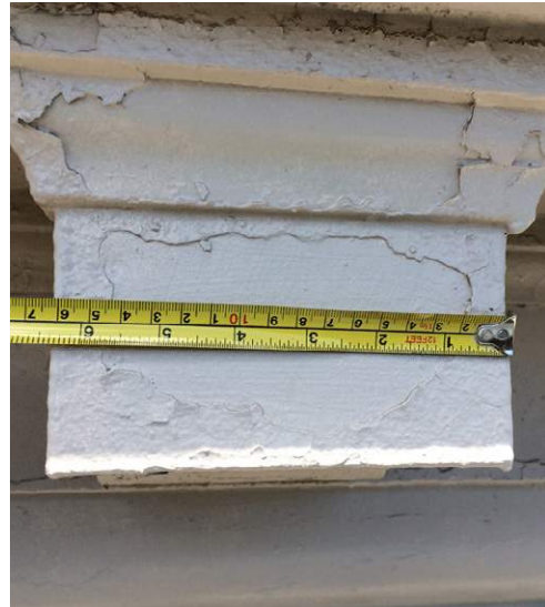
RUSSELL HALL, PAINTED COPPER CORNICE TO BE RESTORED
