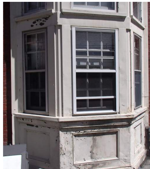
WESTMORLY, PAINTED COPPER WINDOW BAY TO BE RESTORED
