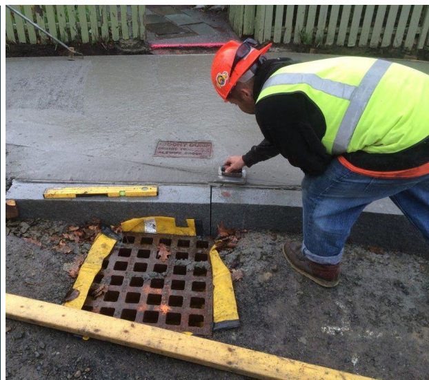
Silt sack installed in a catch basin to manage stormwater pollution during construction
