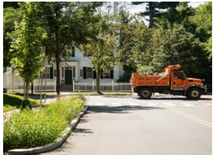
Installation of a rain garden to treat stormwater before it enters the drainage system as part of a sewer separation project.
