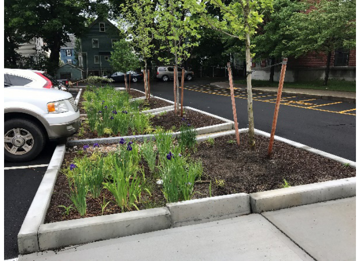
Figure D.5. Tree planters and a bioretention basin are installed in a parking lot of Irving School in Roslindale, Boston. (Source: Boston Water and Sewer Commission (BWSC) and Greenovate City of Boston)
