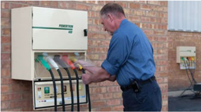
Figure B.7. Emergency generator. (Source: Powertron Solutions)
