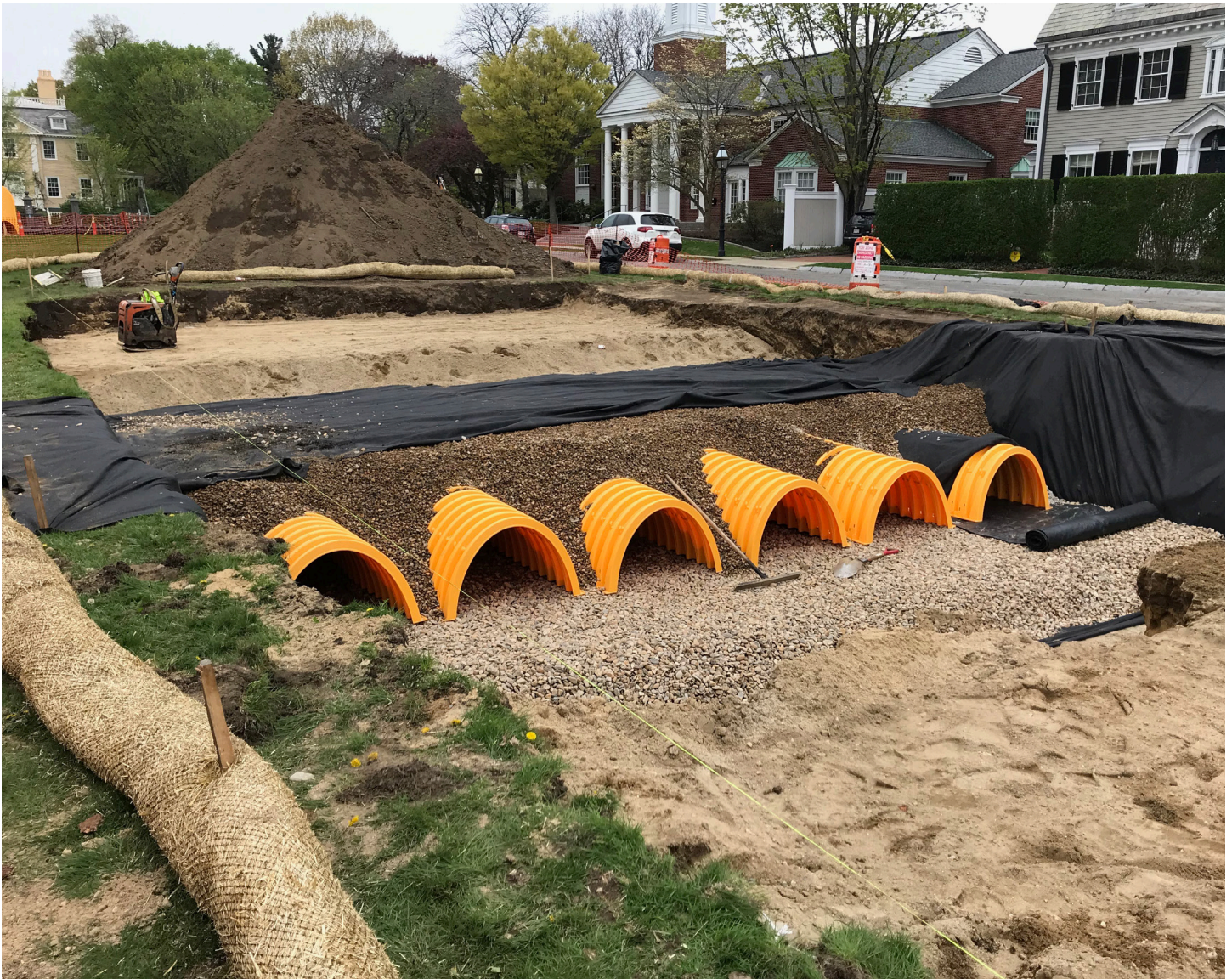
Figure C.12. Subsurface infiltration system to help manage stormwater runoff at Longfellow Park. (Source: City of Cambridge)
