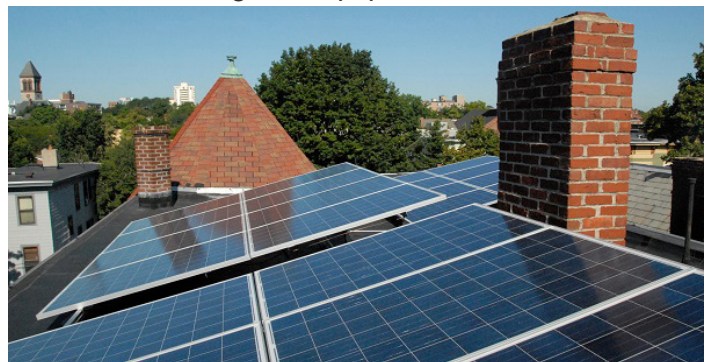
Figure C.13. Solar panels on a pitched roof.
