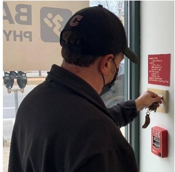
A member of Fire Prevention testing a fire alarm system
