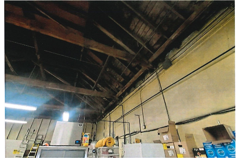
MIDDLE BUILDING EXISTING DETERIORATED ROOF STRUCTURE
