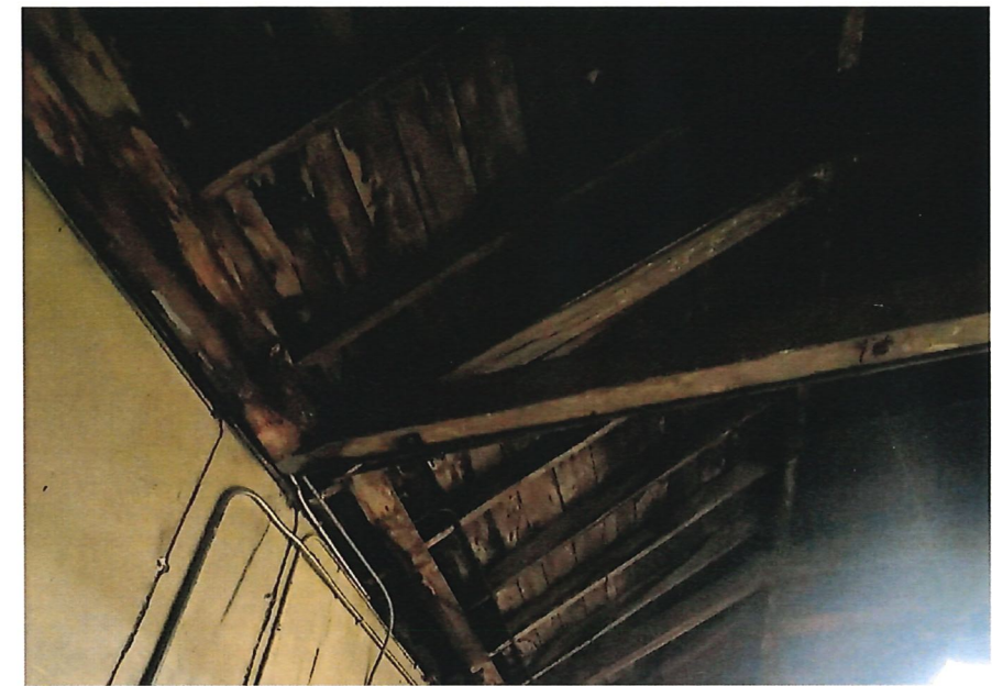
MIDDLE BUILDING EXISTING DETERIORATED ROOF STRUCTURE
