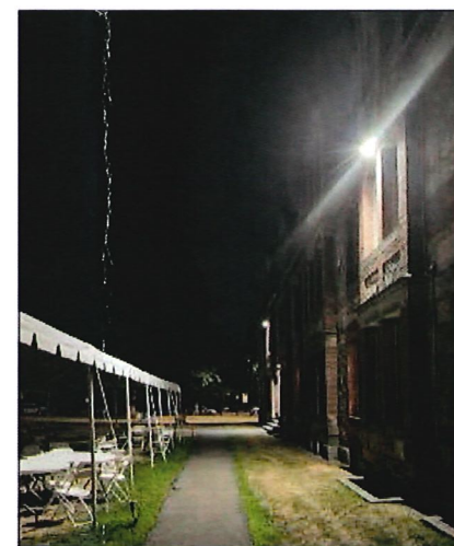
Type C: Building mounted Floodlight (not shown in the plan)
