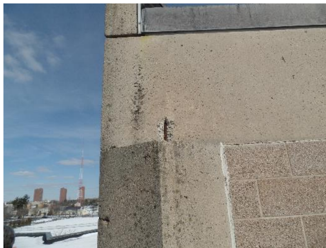
Photo 2: Corroded Reinforcing/Spalled Concrete Cover
