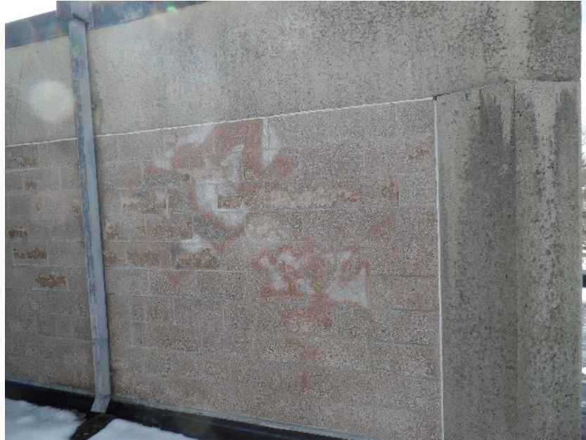
Photo 9: Exterior Masonry Wall - Moisture Damage
