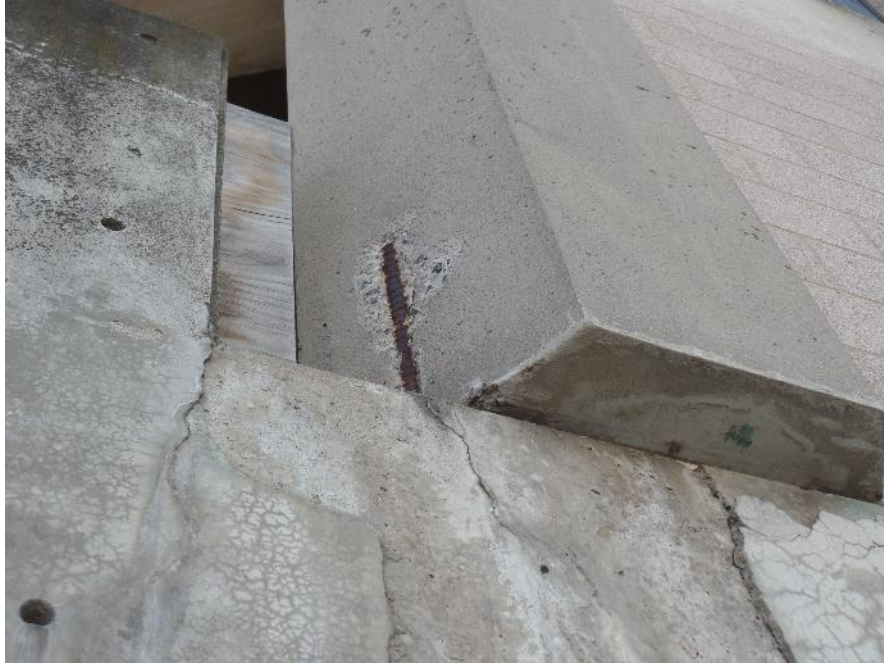
Photo 5: Corroded Reinforcing/Spalled Concrete Cover
