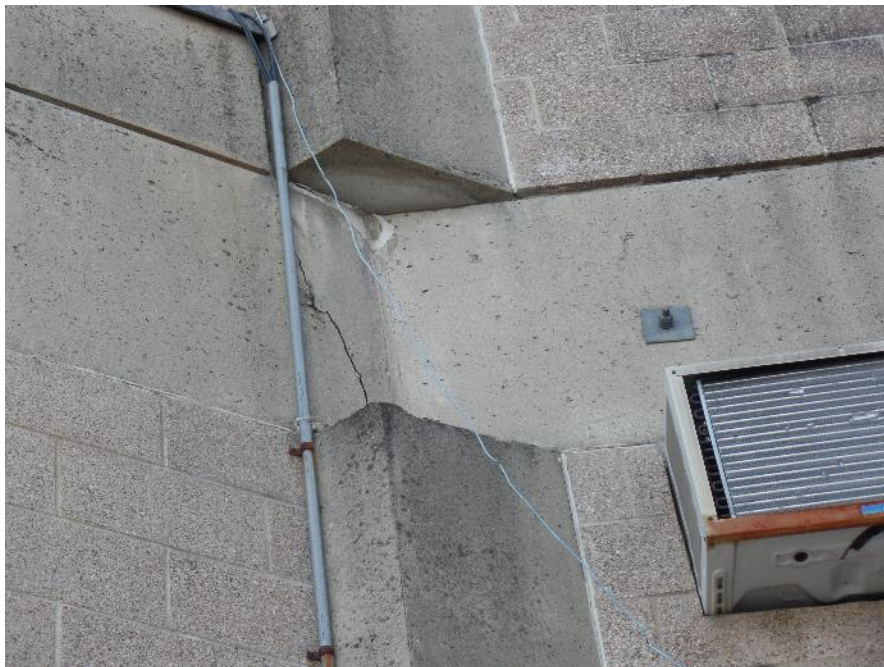
Photo 6: Crack in Concrete Spandrel Beam
