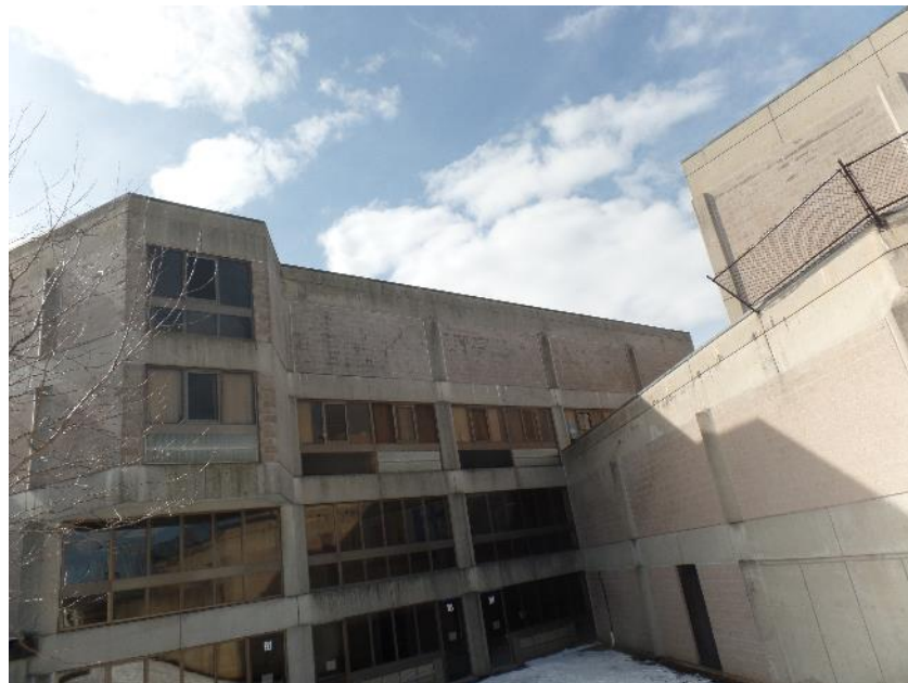
Photo 16: Exterior Masonry Wall - Surficial Damage
