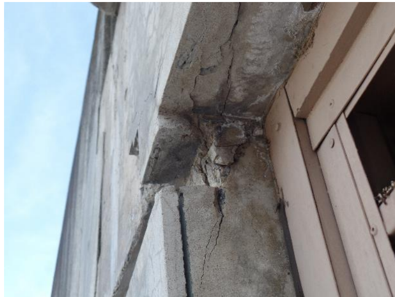
Photo 8: Corrosion/Spalled Concrete Cover and Cracking/Deterioration
