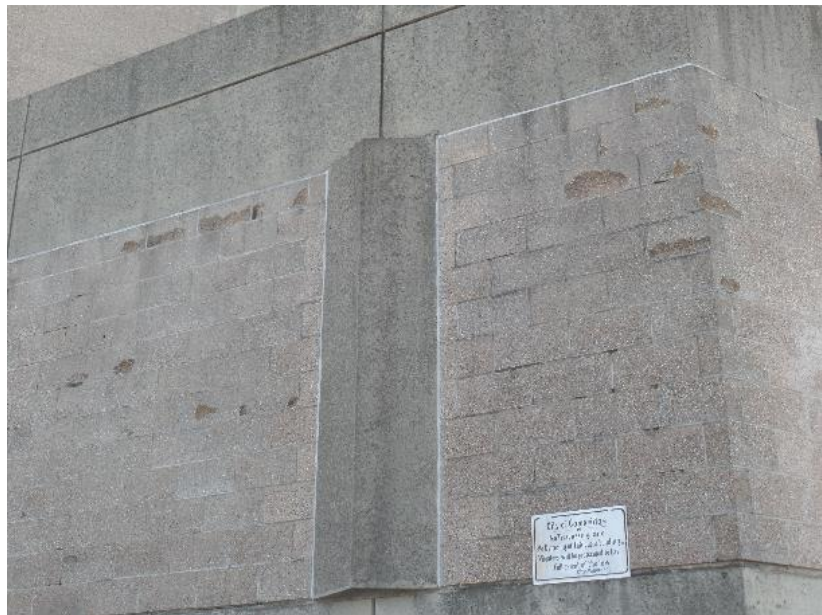
Photo 14: Exterior Masonry Wall - Surficial Damage
