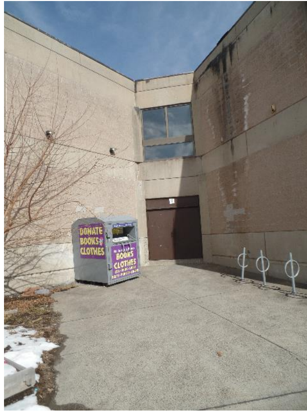
Photo 11: Exterior Masonry Wall - Moisture Damage
