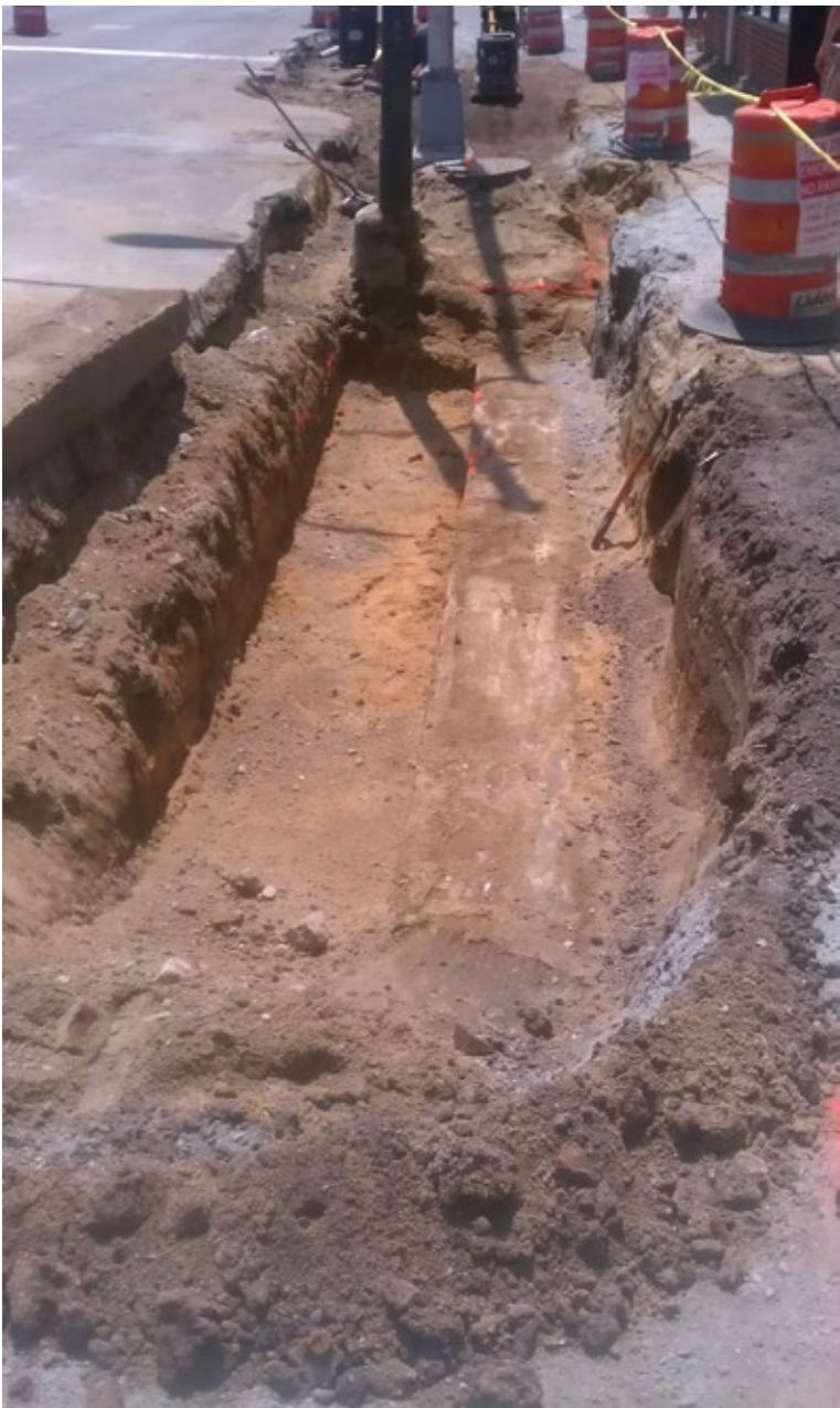
MASS AVE BETWEEN HUDSON ST AND SHEPARD ST
