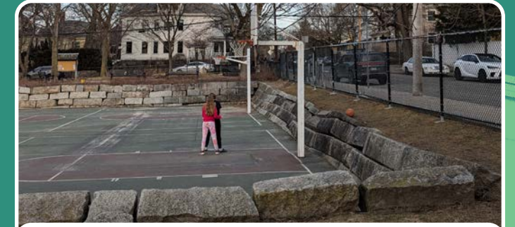
Stabilize slope & address retaining wall failure at Upland Road
