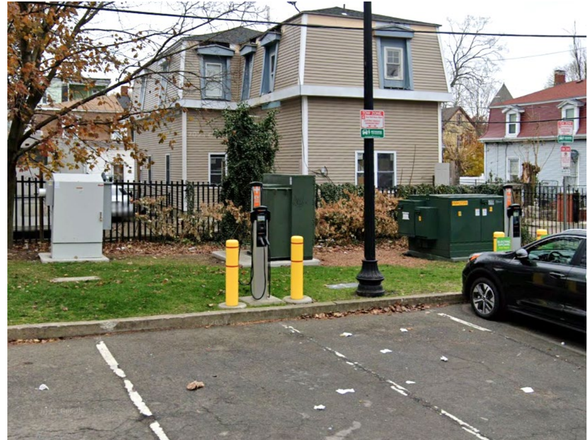
A planned level 3 charger on Hamlet Street in Boston – the three metal cabinets and required setbacks use a lot of land
