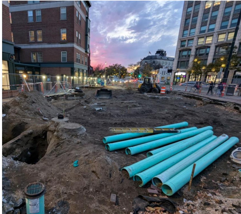
Carl Barron Plaza construction work zone where River St. meets Mass Av.
