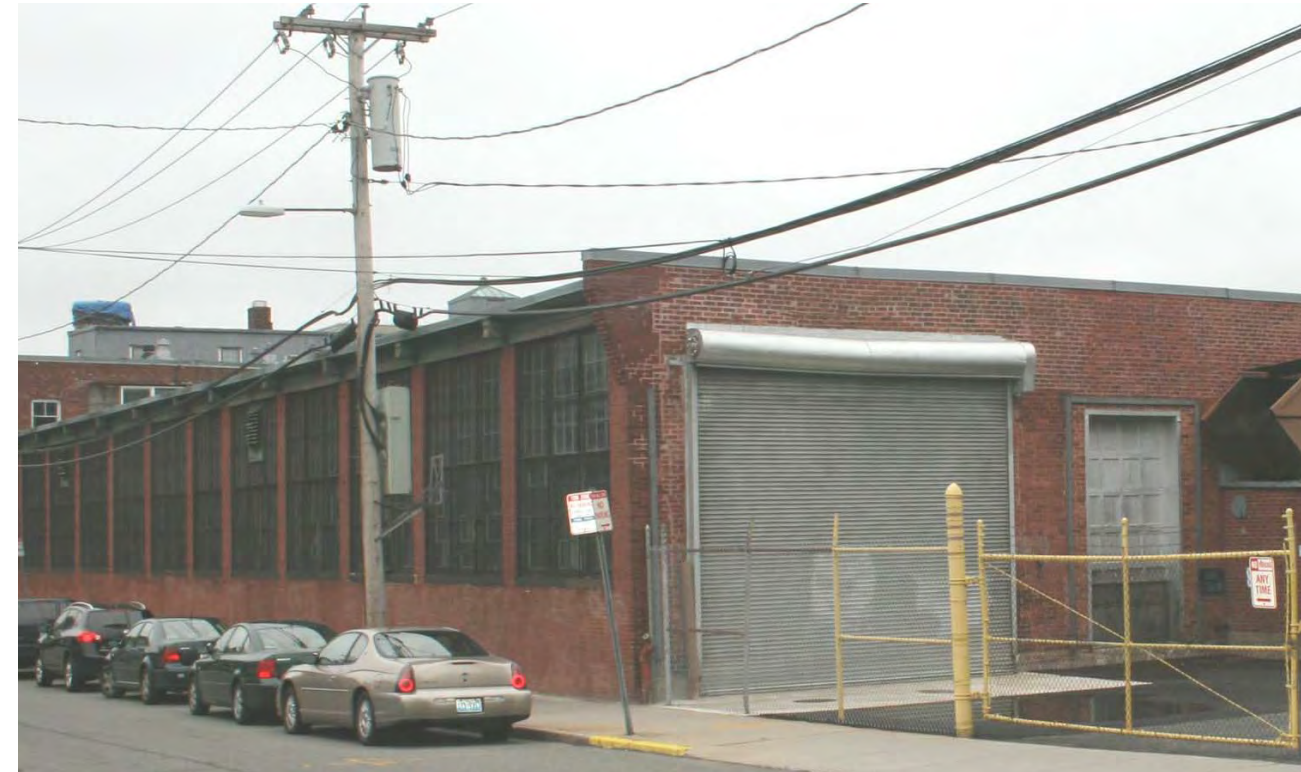
East end of building. These two doors will be replaced with a combination of insulated windows and insulated infill panels to retain the scale of openings.
