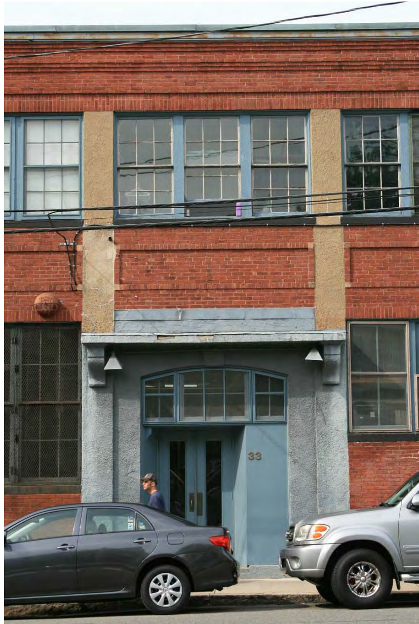
Existing stucco entry lacking in detail and execution is also not accessible to the physically disabled. Entry will be restored to original door design, and made accessible.
