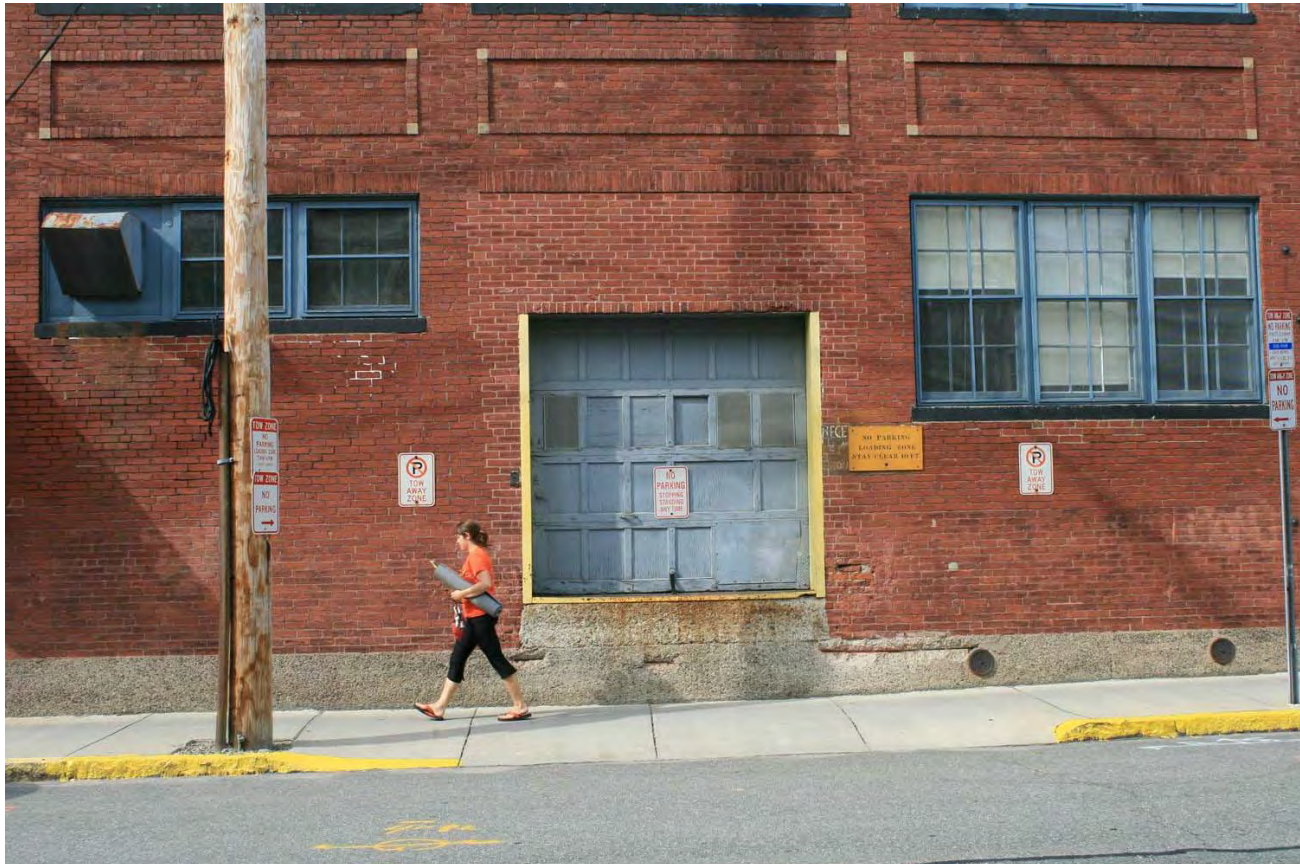
This bay of the building has been adapted over time and no longer bears resemblance to the original design. A new window will replace the garage door. A window will also be inserted to match others to left of garage door.
