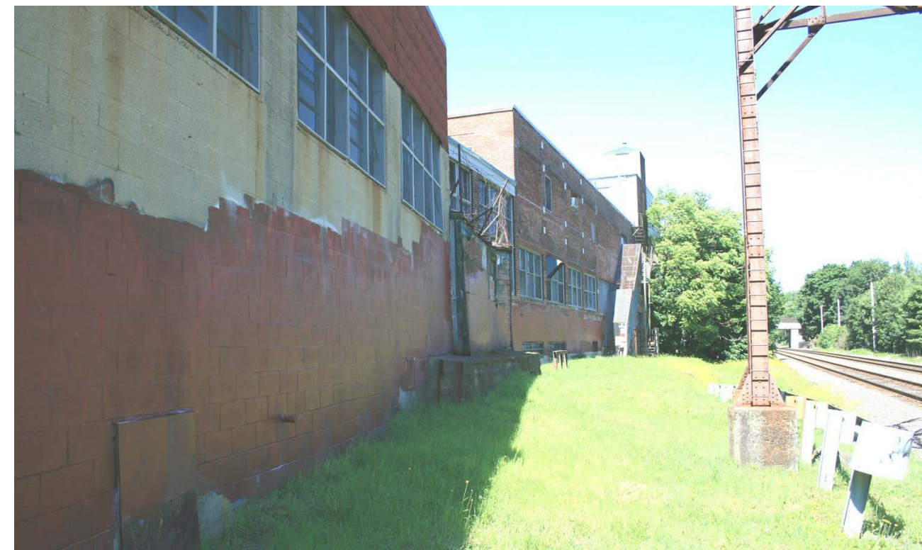
Existing building looking west on rail road right-of-way. Shed and additions that are in poor condition will be removed. Addition above is a concrete block structure that is a more recent addition.
