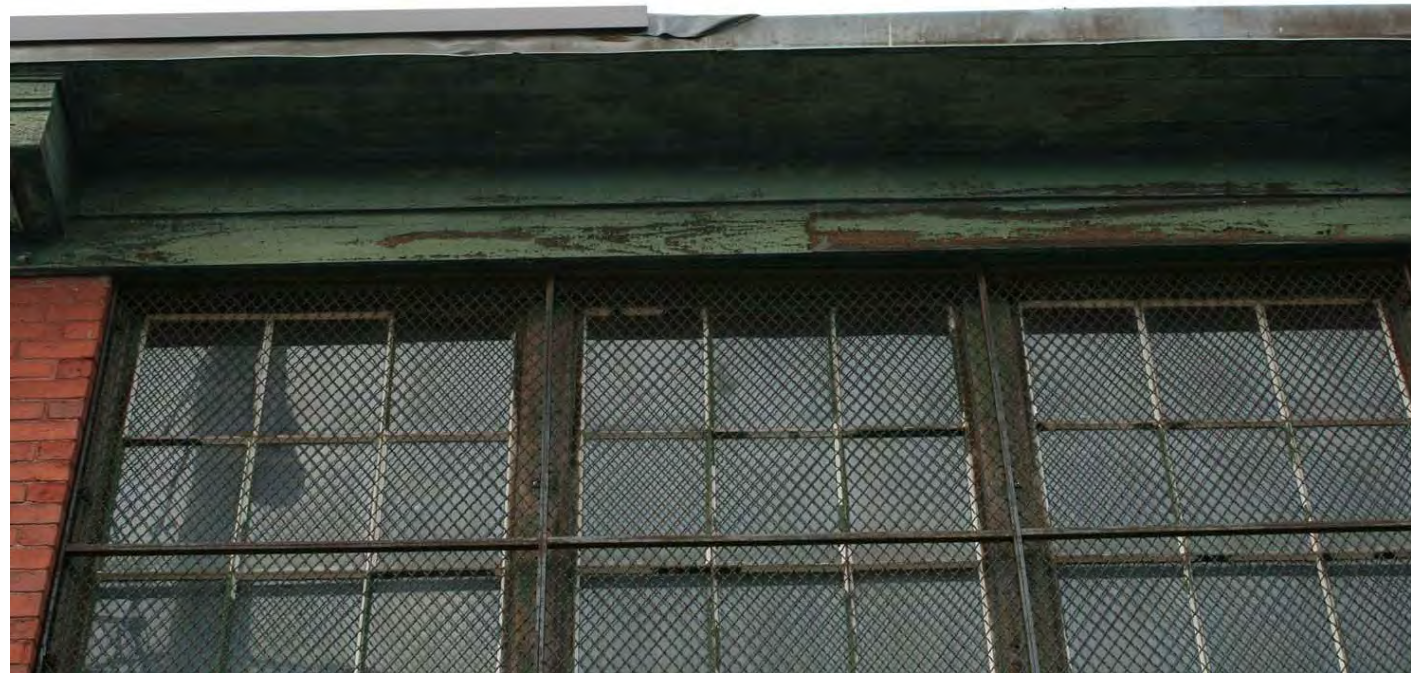
Roof eave requires significant repair. Windows will be replaced with energy efficient sash using similar mullion pattern.
