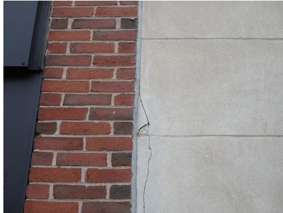
CRACK IN LIMESTONE TO BE REPAIRED WITH PINS AND GROUT
