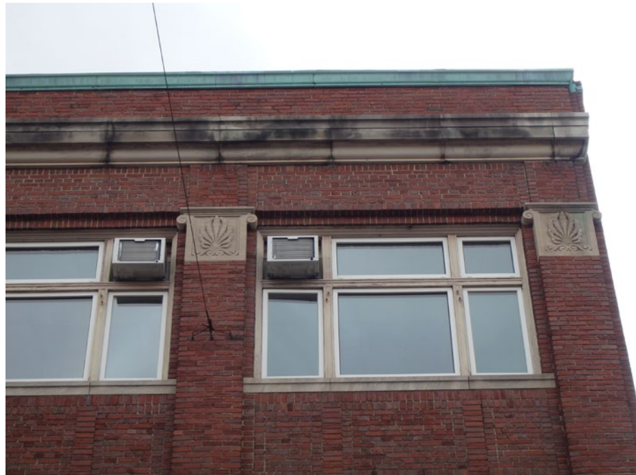
TYPICAL LIMESTONE AND BRICK SOILING
