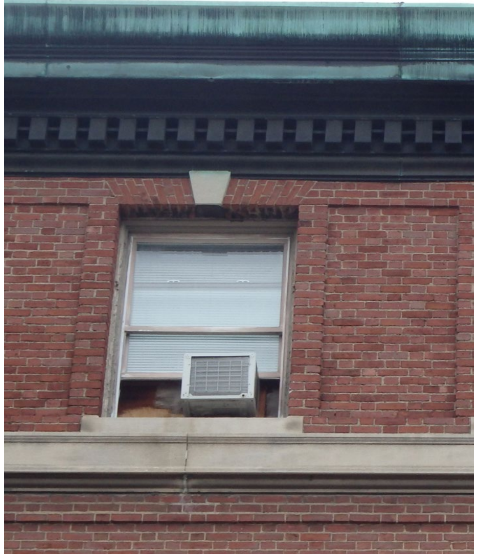
OPEN JOINTS AT LIMESTONE BELT COURSE. COPPER CORNICE TO BE INSPECTED
