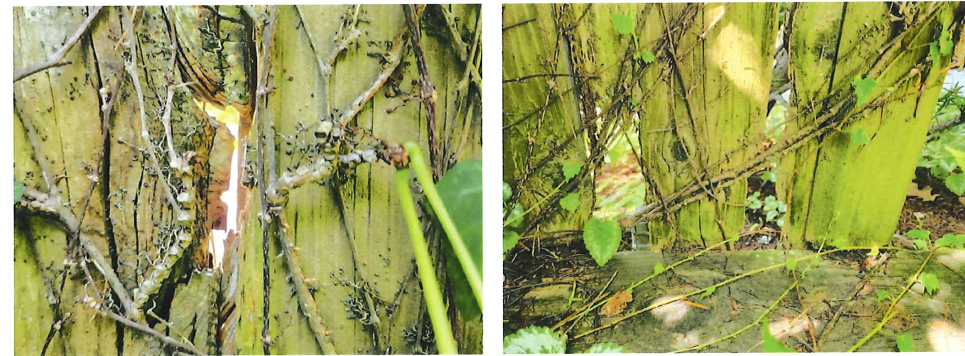
Notes: 1. Large openings are observed throughout the front property line fence. 2. The fence has reached the end of it useful life due to the presence of the large openings which have reduced the structural integrity of the fence.
